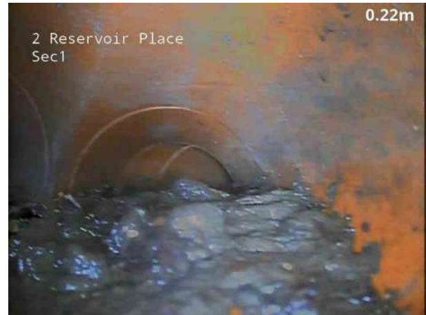
2, 00:00:06, 0.30 m Settled deposits, fine, 50% cross-sectional area loss, change
