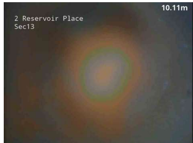
6, 00:00:35, 10.10 m Attached deposits, fouling from 5 o'clock to 7 o'clock, 5% cross-sectional area loss, finish
