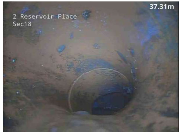
4, 00:02:44, 37.50 m Line deviates down
