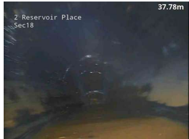
10, 00:03:06, 37.40 m Attached deposits, fouling from 3 o'clock to 9 o'clock, 20% cross-sectional area loss, finish
