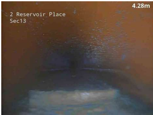
3, 00:00:21, 4.30 m Attached deposits, fouling from 5 o'clock to 7 o'clock, 10% cross-sectional area loss, change, Scale
