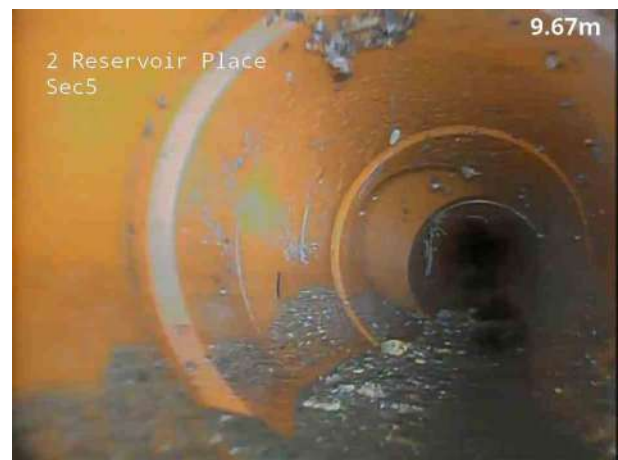
4, 00:00:37, 9.70 m Line deviates right
