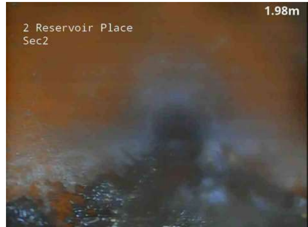
2, 00:00:43, 2.00 m Settled deposits, fine, 5% cross-sectional area loss, change
