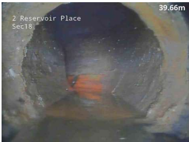
17, 00:04:59, 40.90 m Finish node, manhole, reference: MH1, Small blockage within MH1
