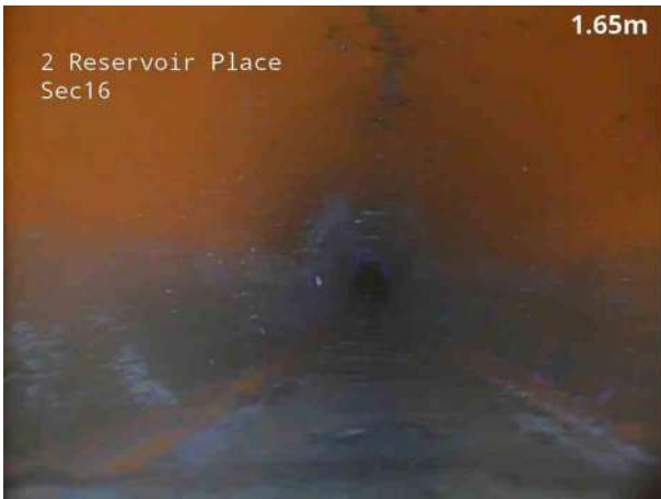
3, 00:00:20, 1.70 m Settled deposits, other, 5% cross-sectional area loss, finish
