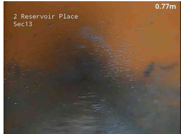
2, 00:00:11, 0.80 m Attached deposits, fouling from 5 o'clock to 7 o'clock, 5% cross-sectional area loss, start, Scale
