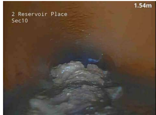
2, 00:00:14, 1.60 m Attached deposits, fouling from 5 o'clock to 7 o'clock, 25% cross-sectional area loss
