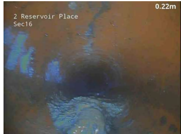
2, 00:00:09, 0.30 m Settled deposits, other, 5% cross-sectional area loss, start
