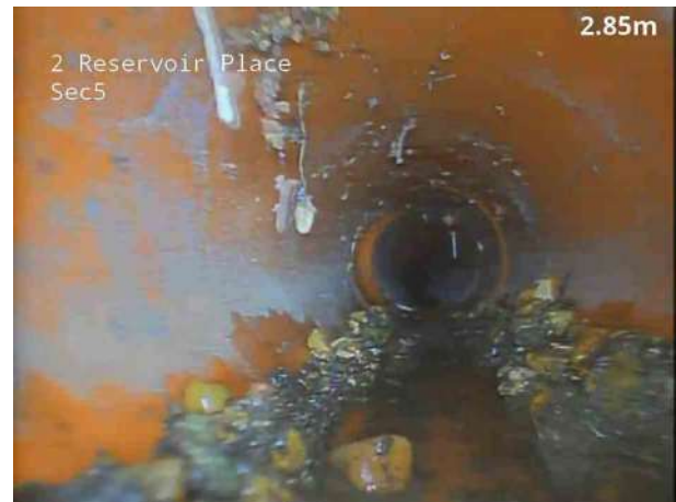
2, 00:00:19, 2.80 m Settled deposits, coarse, 10% cross-sectional area loss
