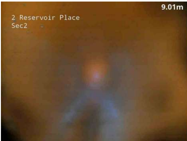
3, 00:01:16, 9.00 m Settled deposits, fine, 5% cross-sectional area loss, finish
