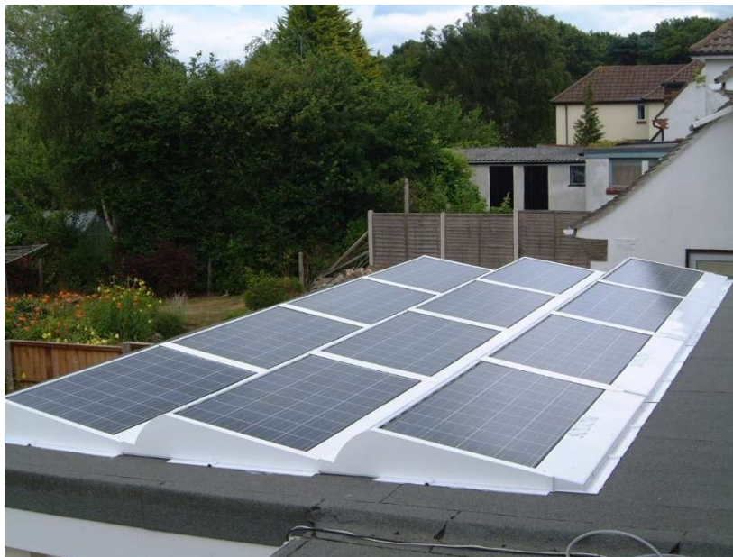
Figures 4: Solar PV installation on a flat roof
