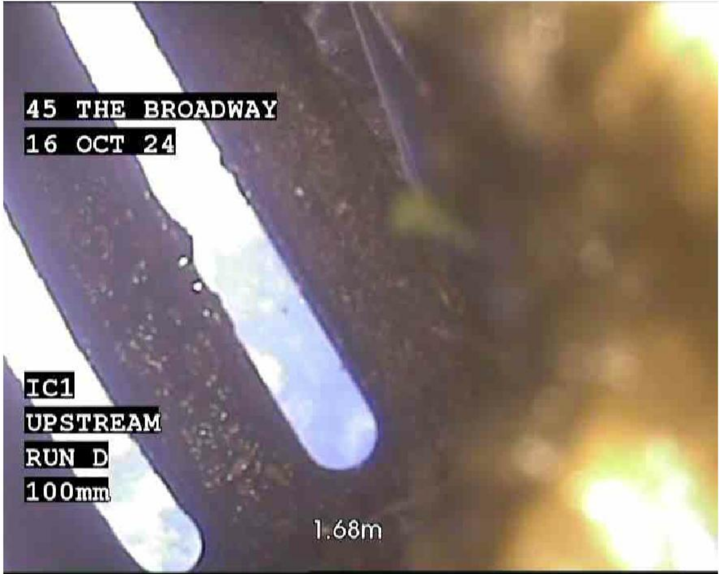
1, 00:00:18, 1.68 m Finish node, manhole, reference: RUN D, At aco drain
