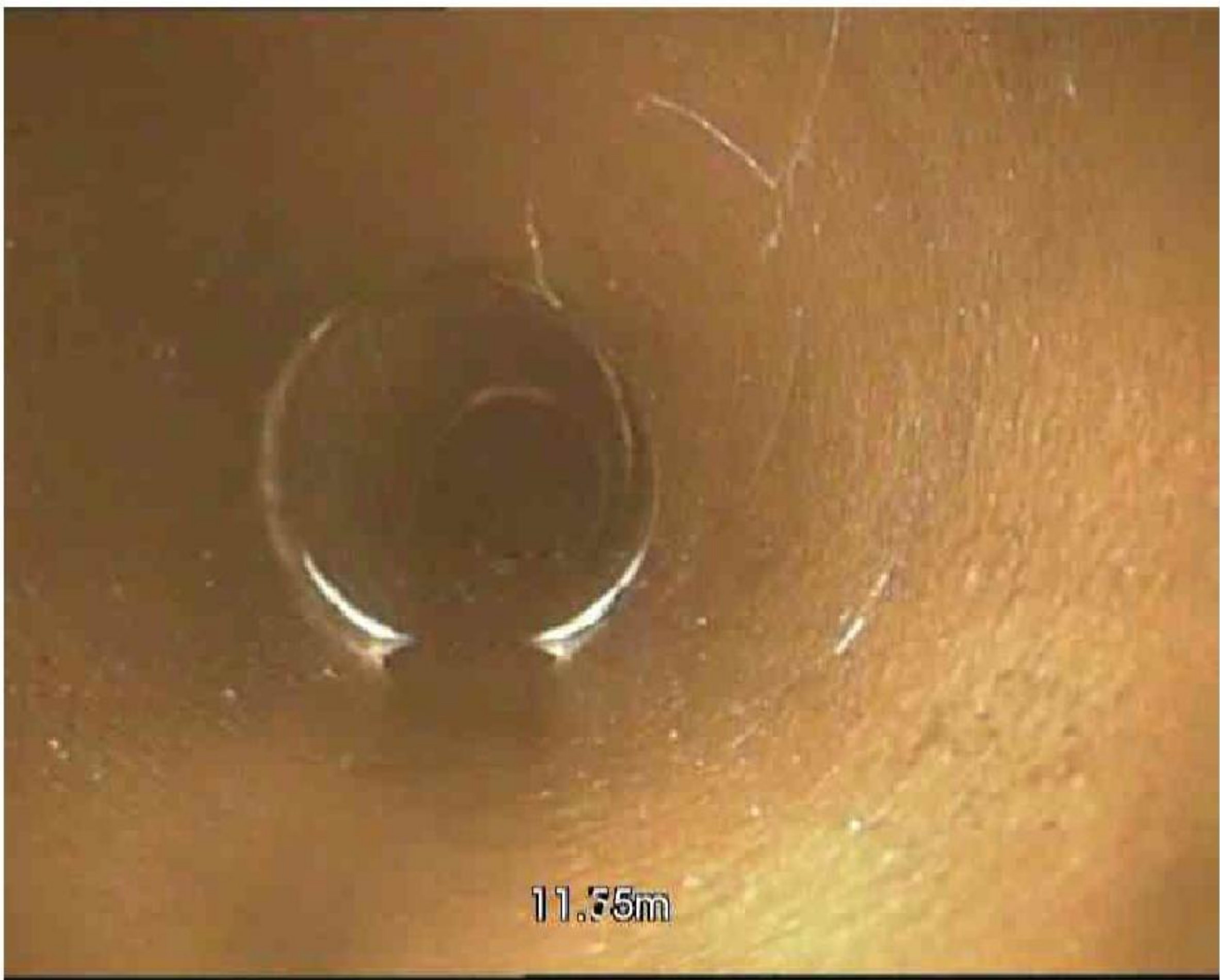
2, 00:01:28, 11.55 m Crack, longitudinal at 01 o'clock
