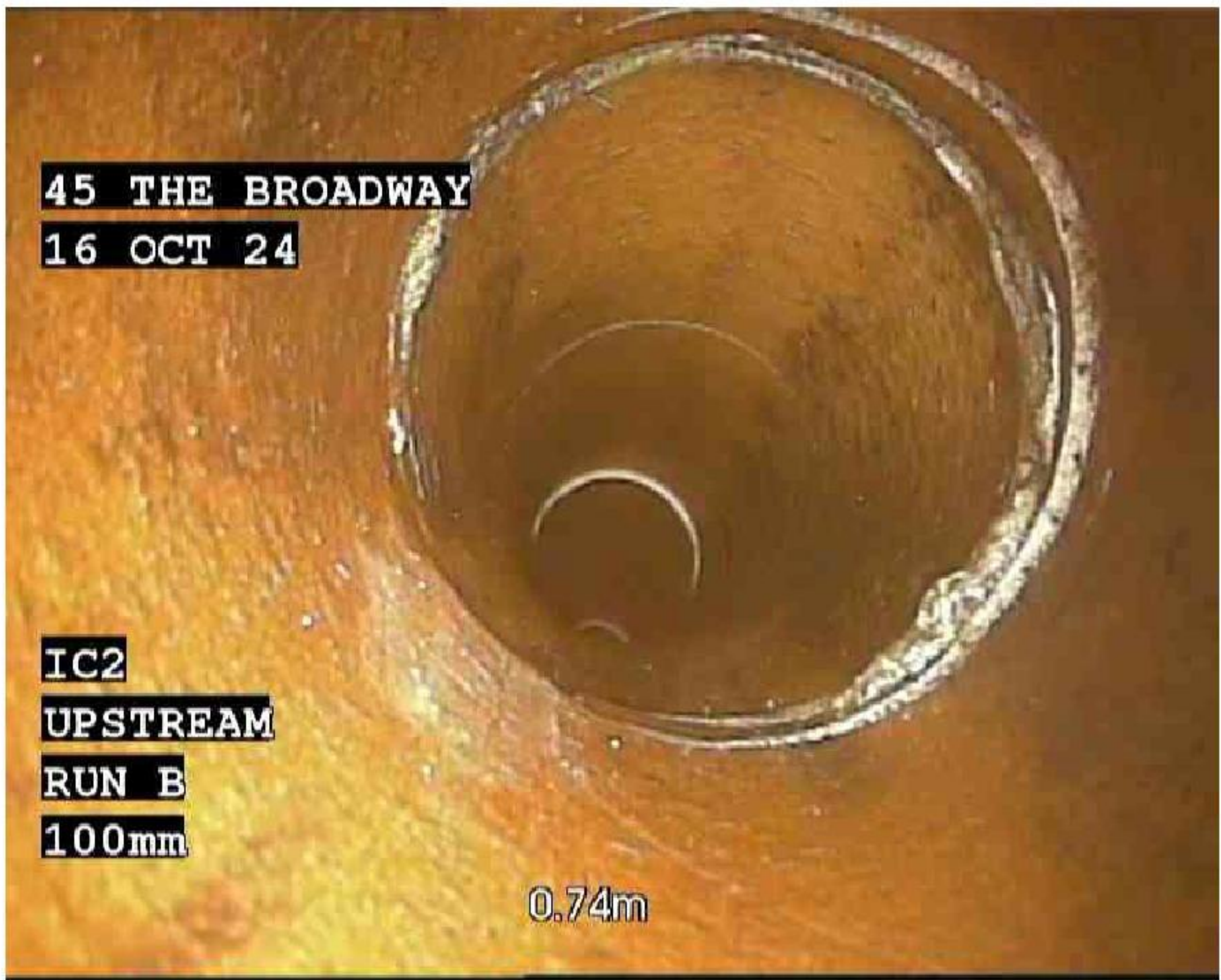
1, 00:00:07, 0.74 m Crack, circumferential at joint from 11 o'clock to 6 o'clock
