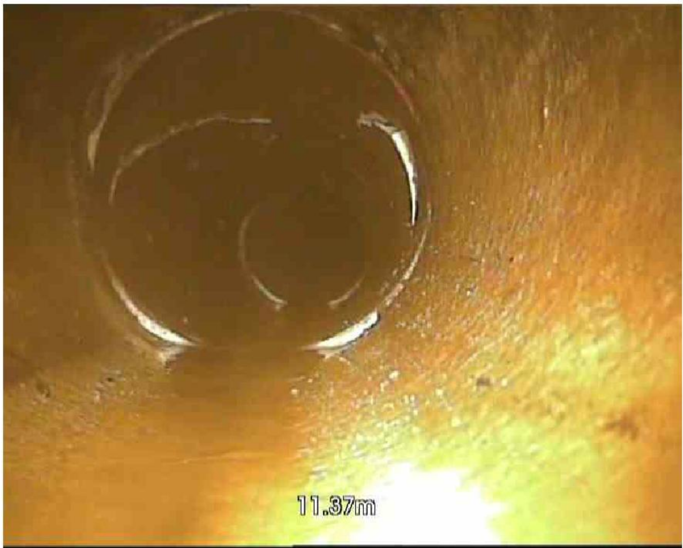
1, 00:01:25, 11.37 m Broken pipe at joint from 9 o'clock to 3 o'clock
