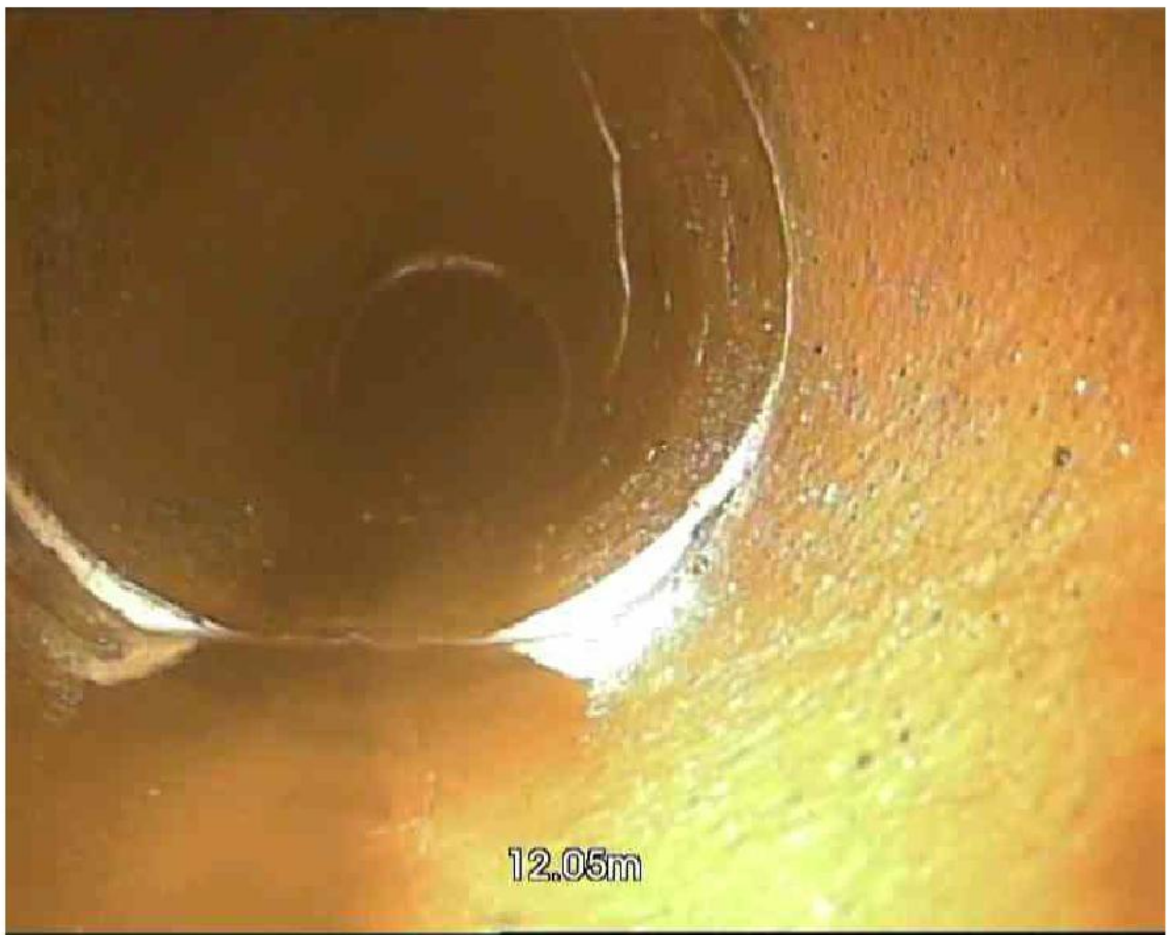
3, 00:01:30, 12.05 m Crack, circumferential at joint from 1 o'clock to 5 o'clock
