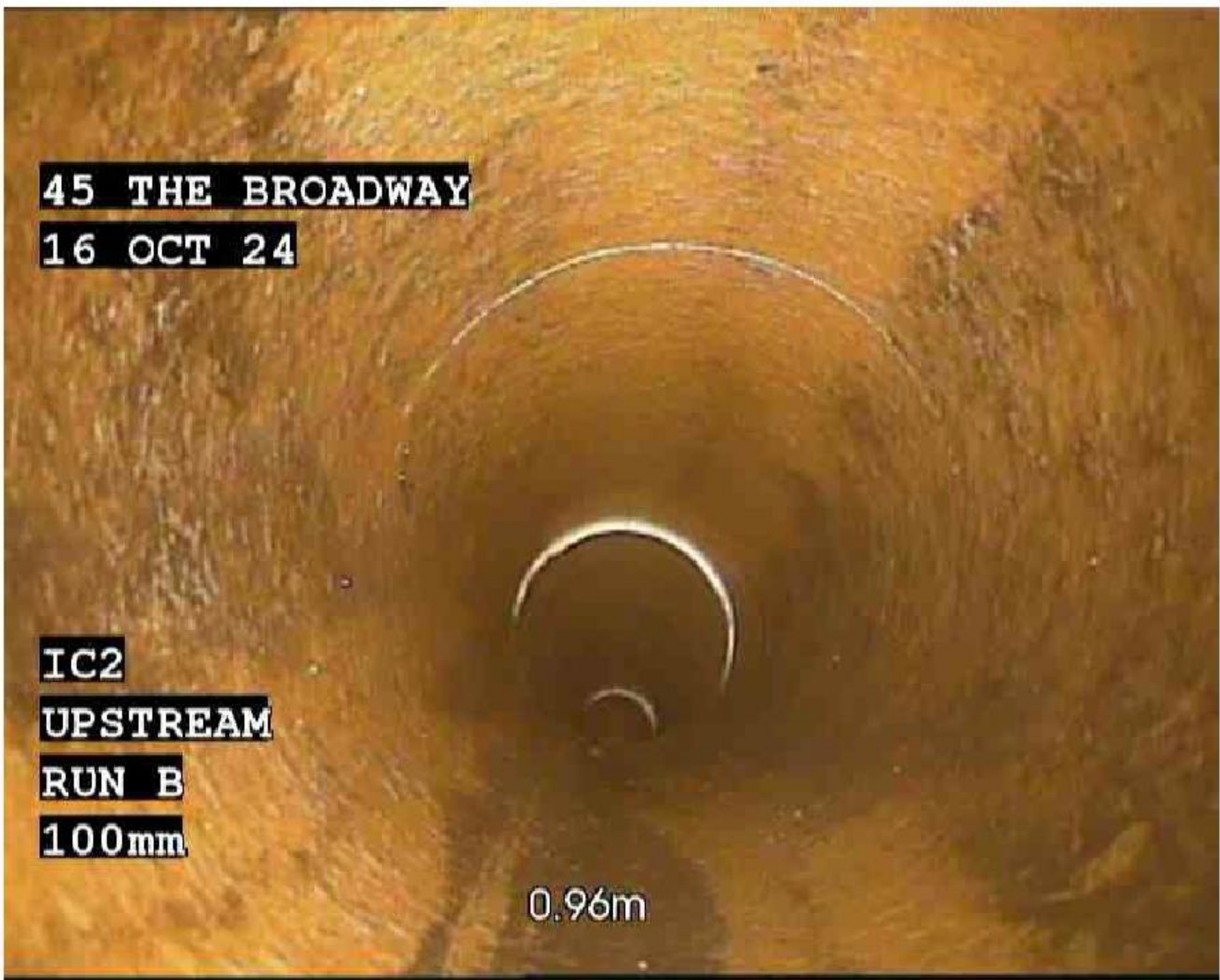
2, 00:00:09, 0.96 m Crack, circumferential at joint from 10 o'clock to 2 o'clock
