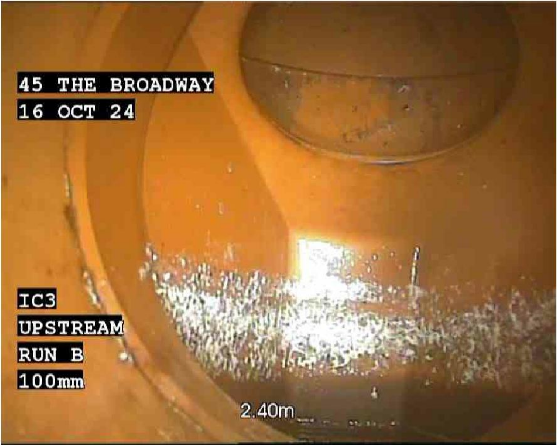
1, 00:00:19, 2.36 m Finish node, manhole, reference: IC3-B, At foul gully (sinks)
