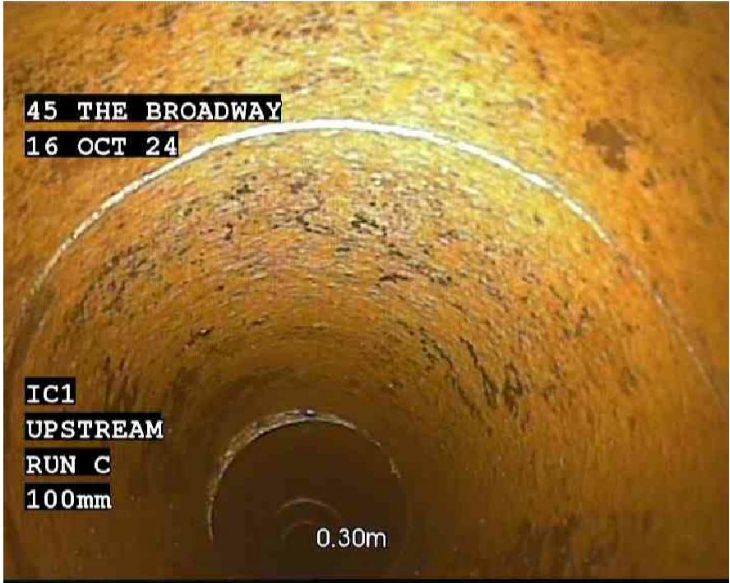
1, 00:00:01, 3.00 m Crack, circumferential from 09 o'clock to 03 o'clock
