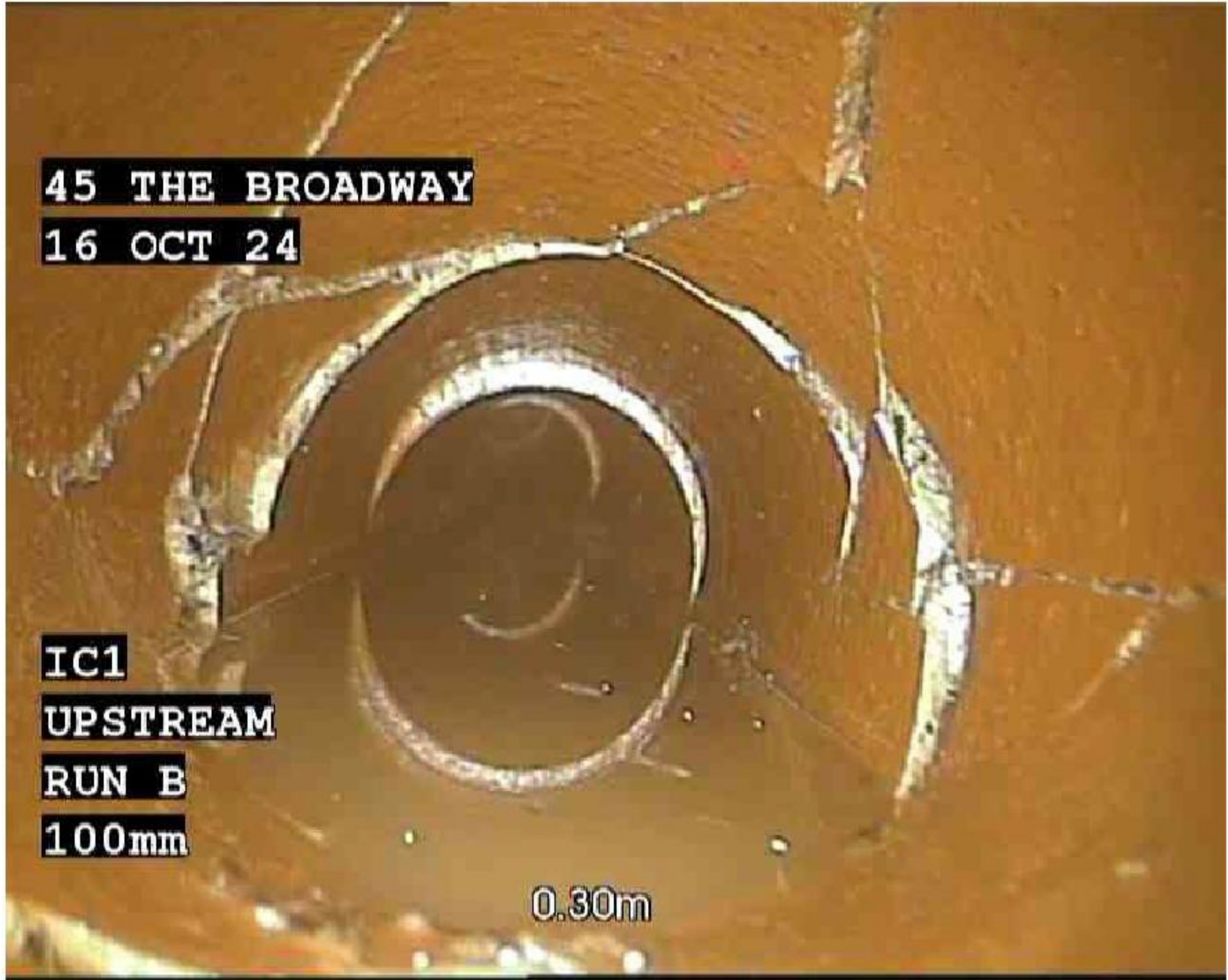
1, 00:00:01, 0.30 m Fractures, multiple at joint from 7 o'clock to 5 o'clock
