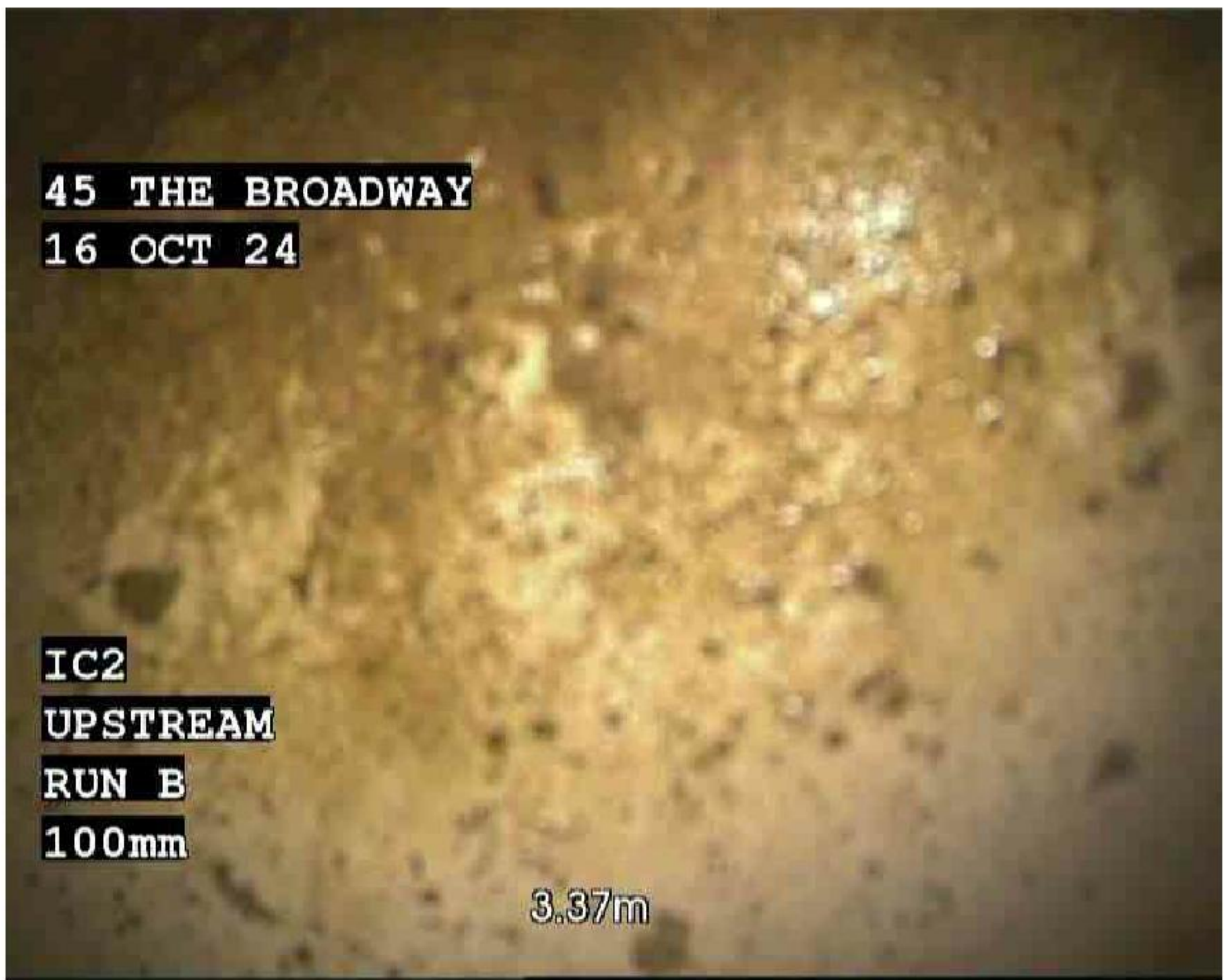
3, 00:00:27, 3.37 m Survey abandoned, Redundant - capped off
