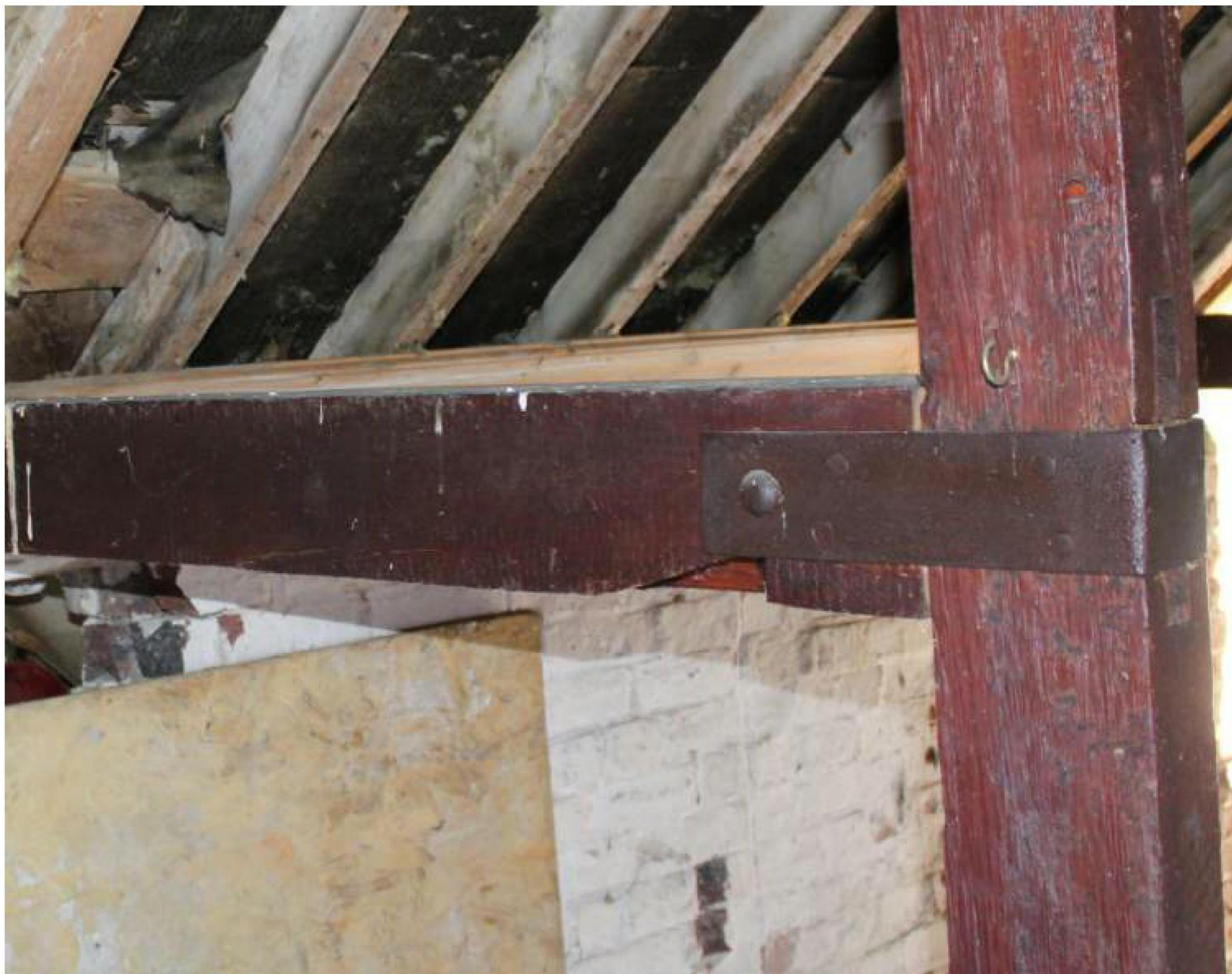
Figure 10 Exposed half joint on Truss 3.
