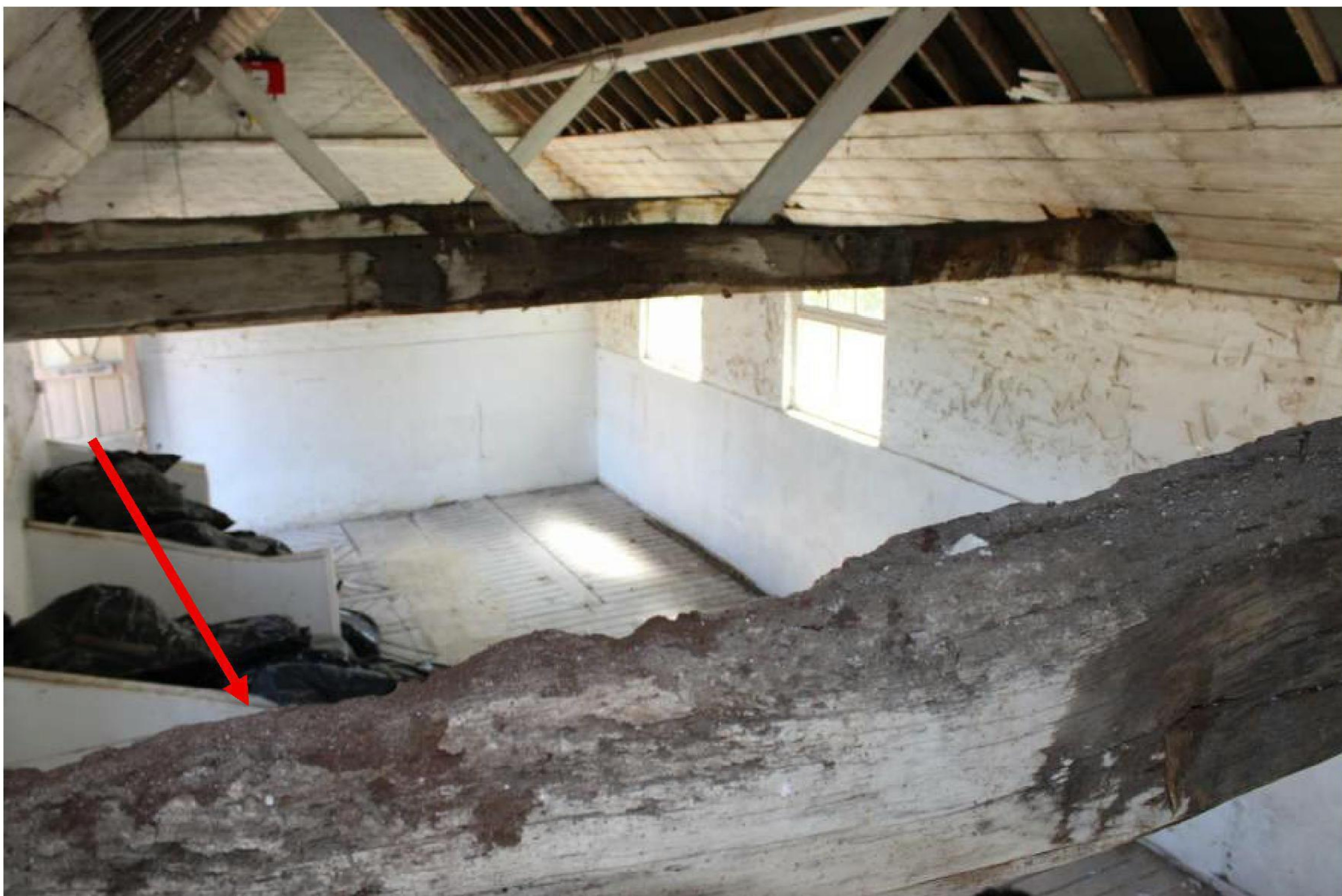
Figure 14 Top surface decay on the north side of the bottom chord of Truss 7 (as denoted by red arrow, Truss 5 is located furthest away in this photo). Some sarking boards are present on the roof.
