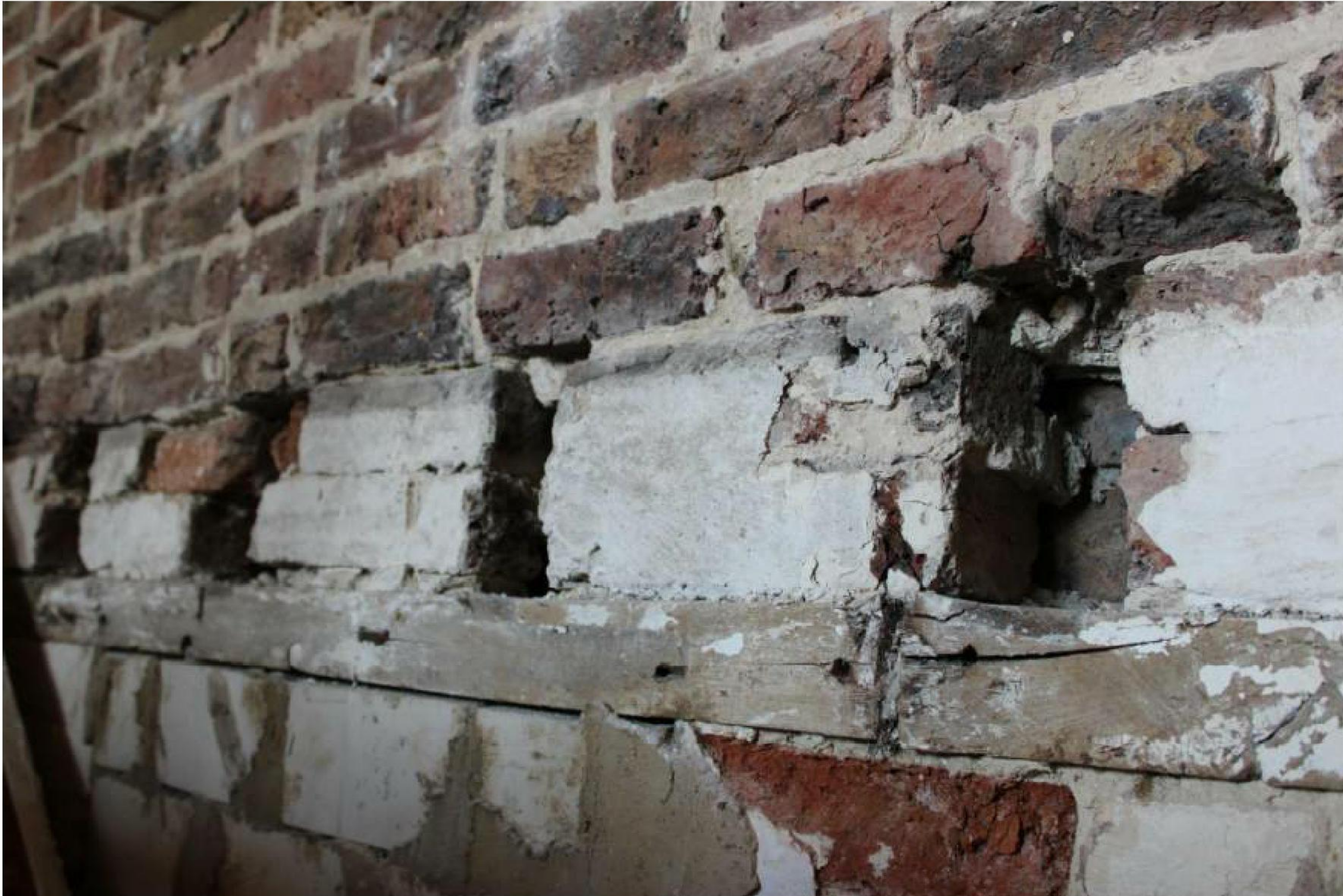
Figure 4 Bricks at joist bearing locations in poor condition.
