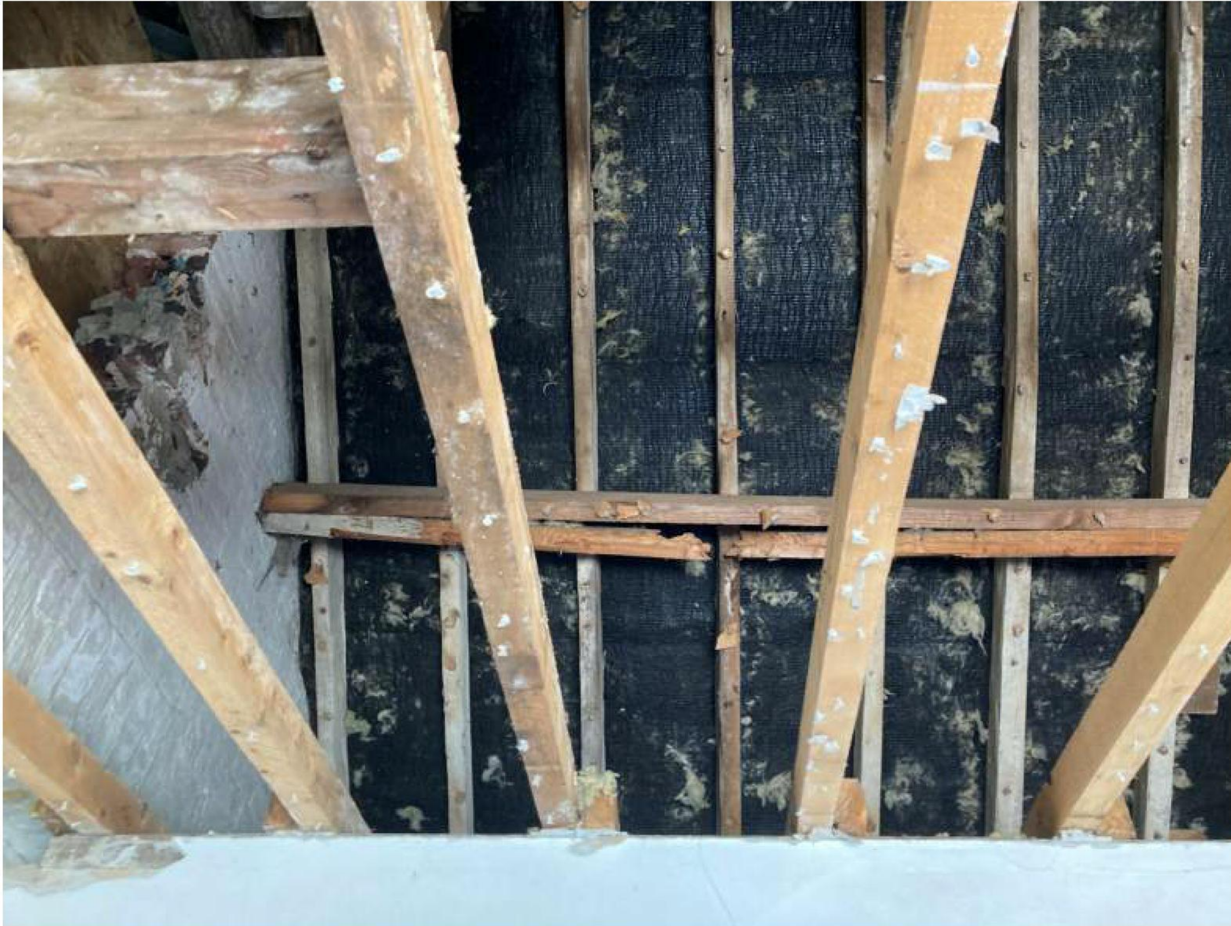
Figure 12 Broken purlin with additional purlin alongside in South Range East.
