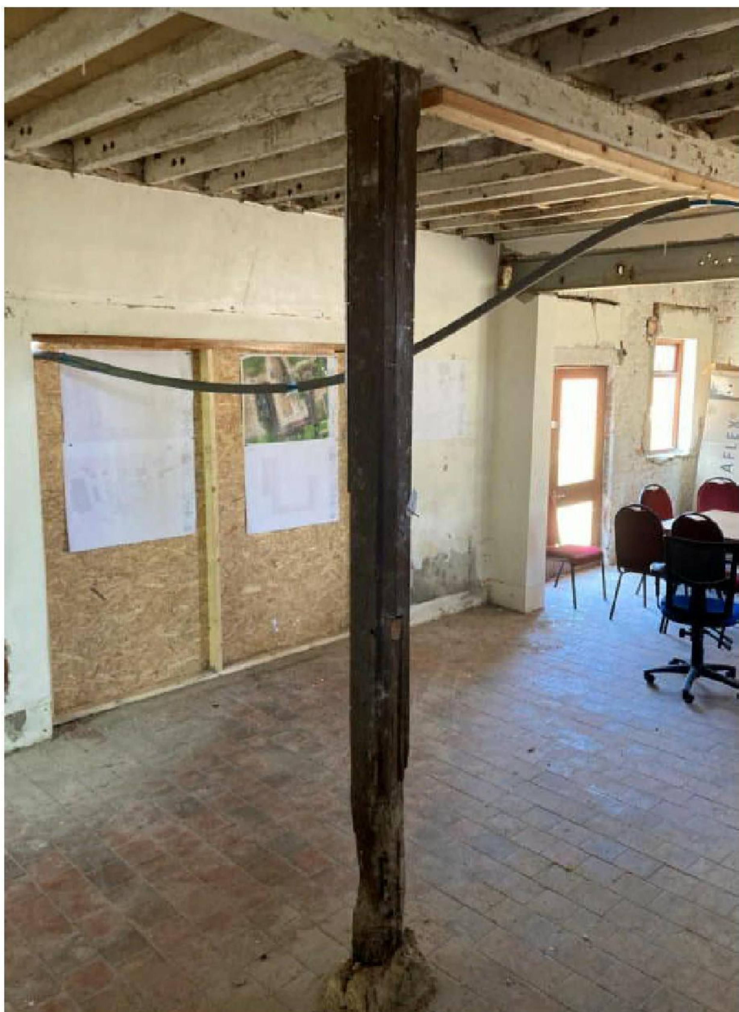
Figure 5 Significant decay at bottom section of timber column.
