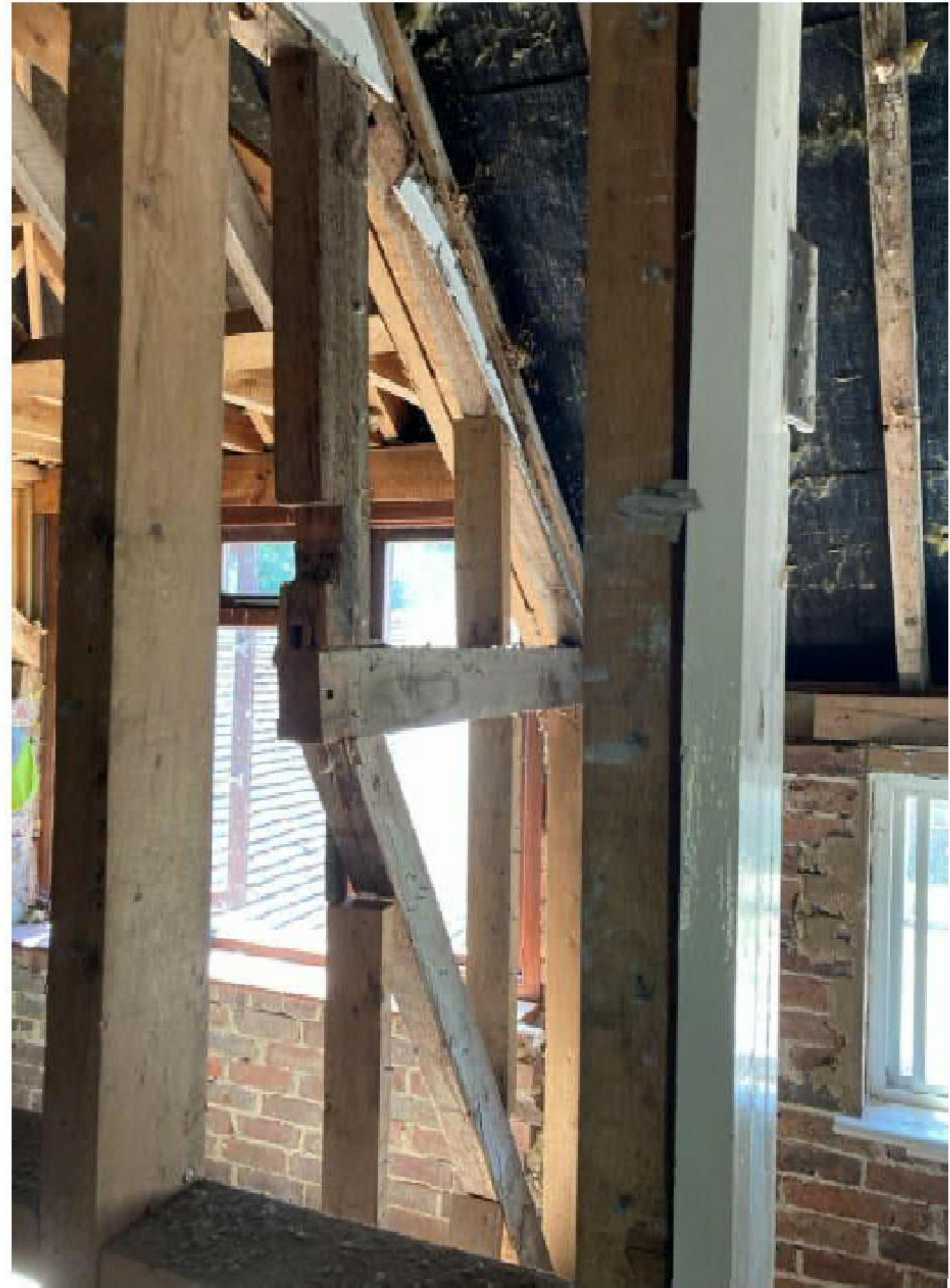
Figure 9 Bottom section of the west timber post removed on Truss 1.
