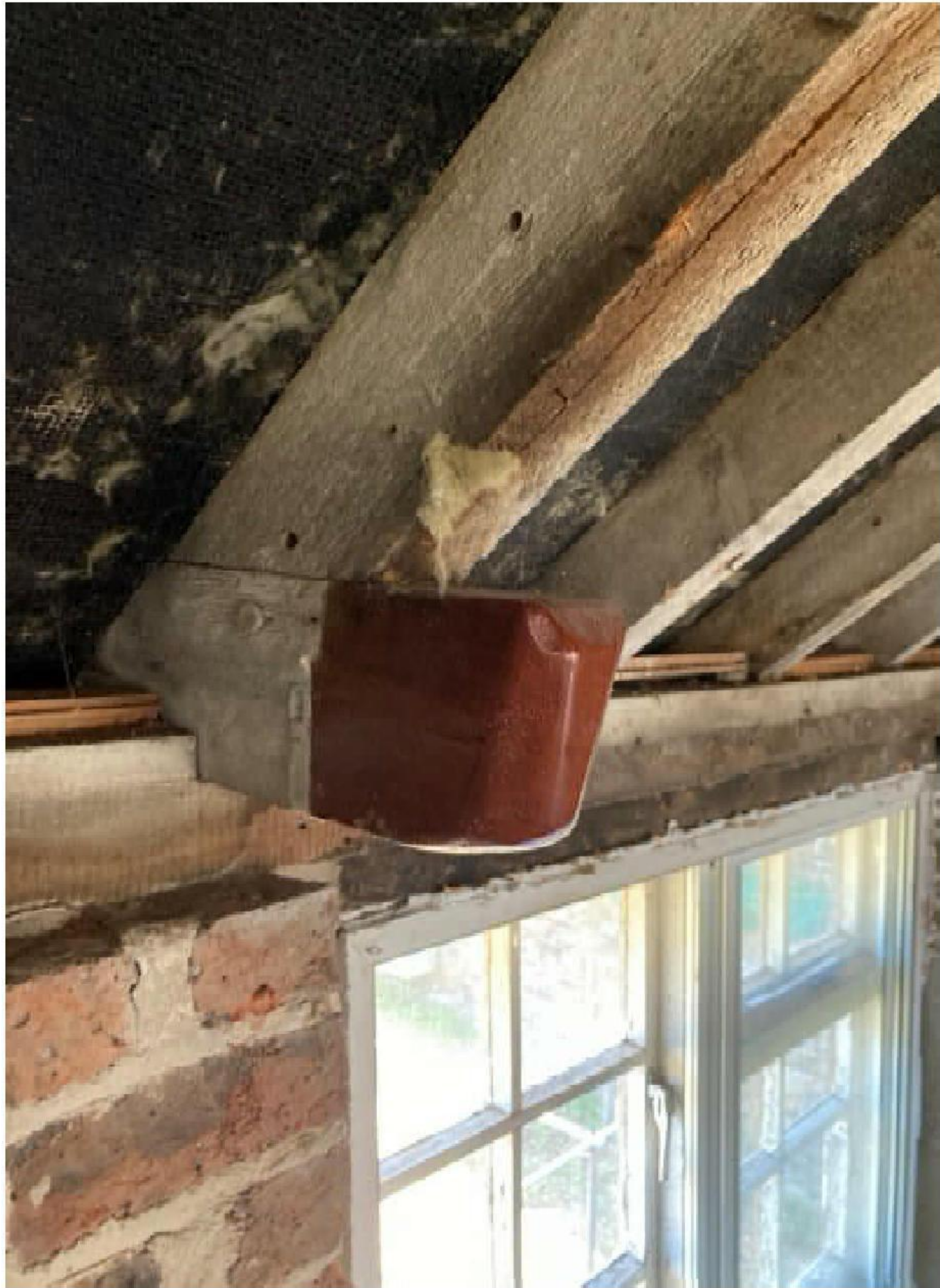
Figure 8 Collar tie removed on Truss 1.
