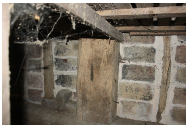
Plate 17. Taper burn mark at the base of the intermediate post in Truss D.
