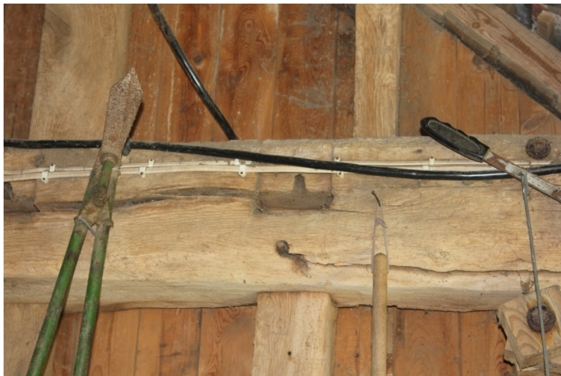
Plate 21. Empty haunched tenon joints in the end girt of Truss A.
