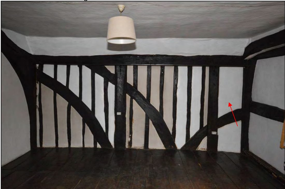
Plate 8: The northeast wall of bay 3 at first floor level on the interior, the low foot-brace to the southeast accommodates a former shuttered opening above it (red arrow, see also Figure 8)
