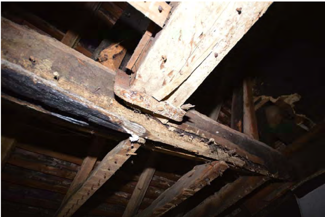
Plate 28: The stirrup strap at the junction of the flying plate and the girder
