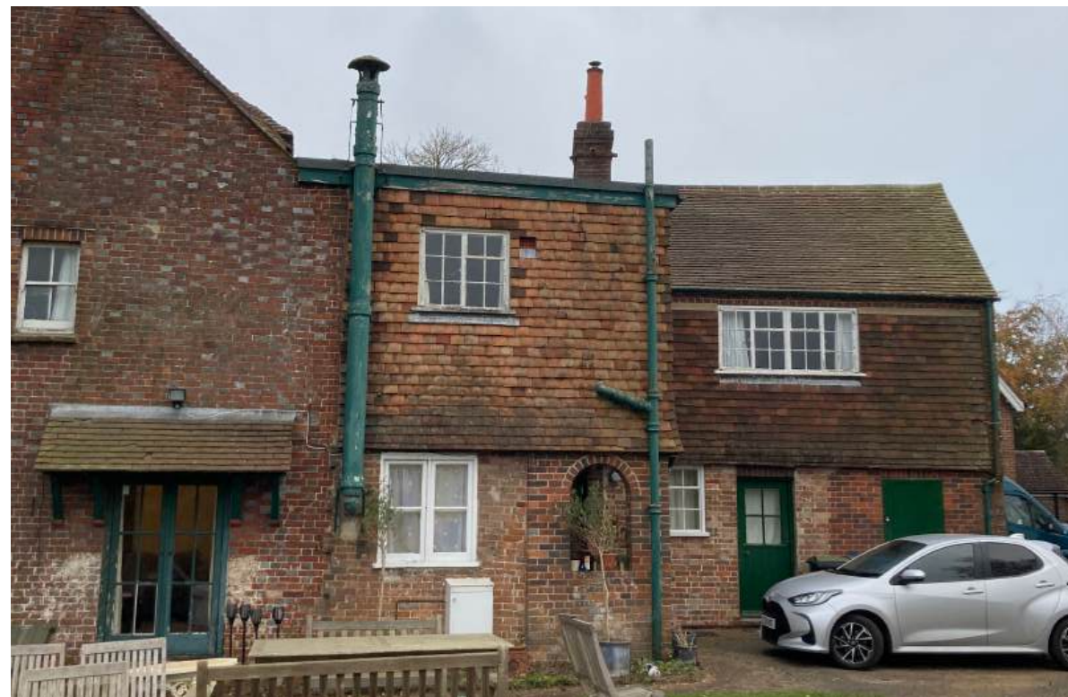
Modern pipes and soil vent pipes to be rationalised and intrernalised.
