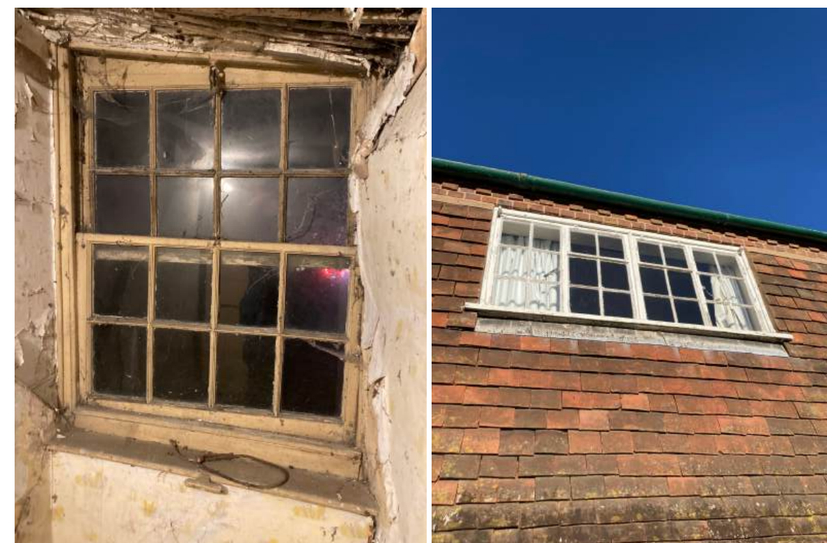
Example of decayed historic window to be replaced (left) and 1950s window to be replaced (right).
