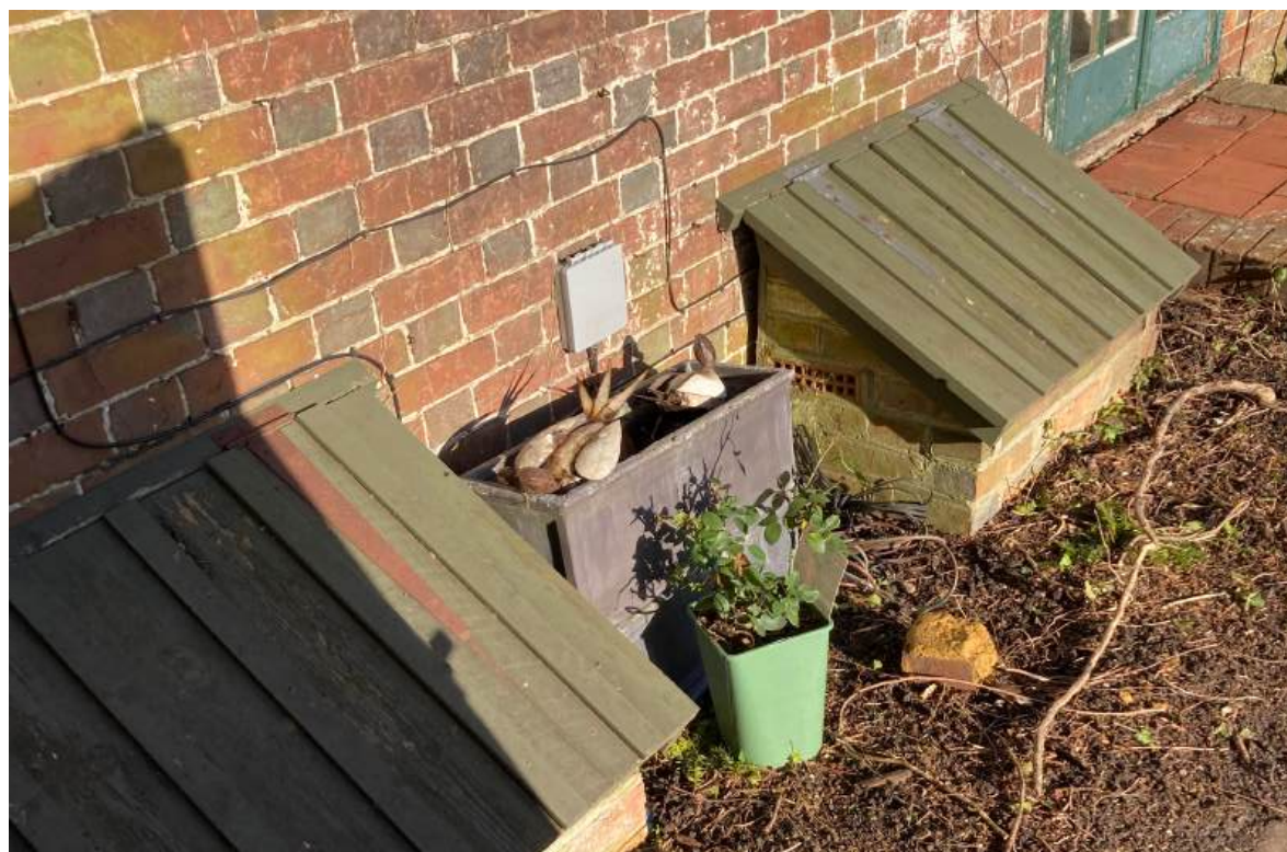
Modern cellar windows' covers to be replaced.
