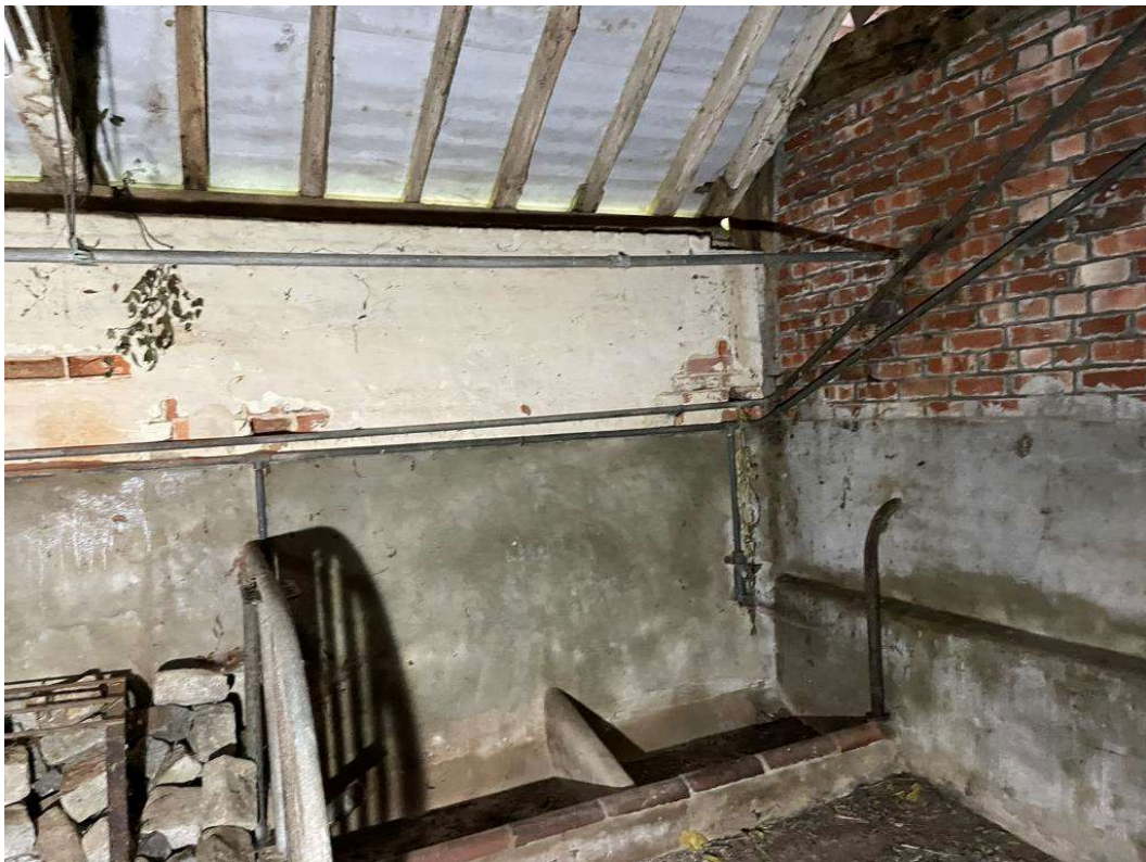
View on front wall of brick barn showing walls and local damage to brickwork
