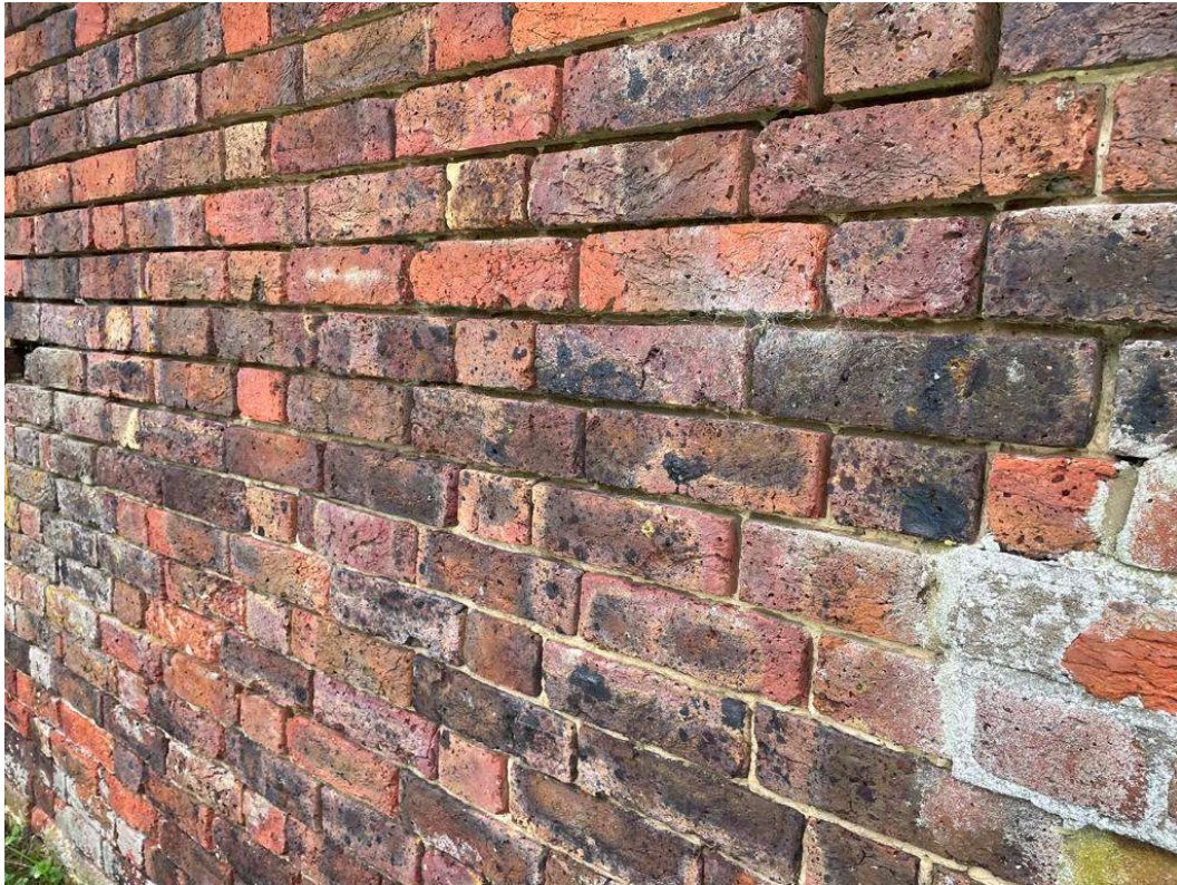
Detailed view on typical arear of front wall brickwork showing mortar recession
