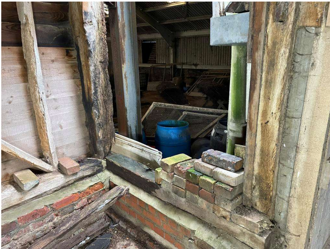
View on rear right corner showing weather damage and decay to corner post and sole plates.
