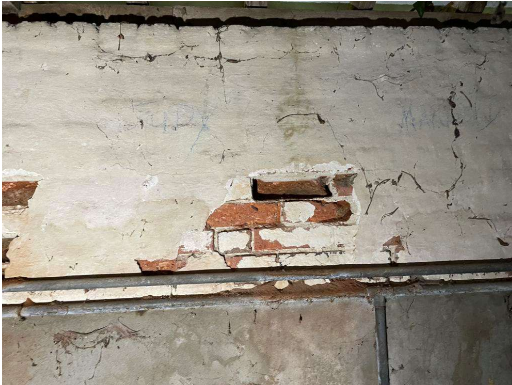
Detailed view on front wall showing eroded bricks
