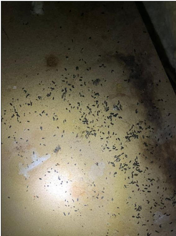
Photograph 1: Mouse droppings in loft.
