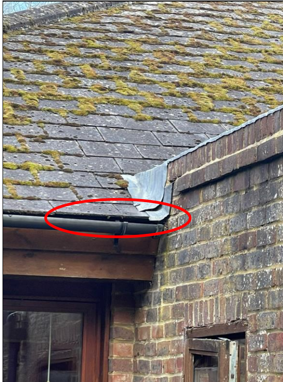
Photograph 13: Raised flashing and gap between roof tiles and guttering.
