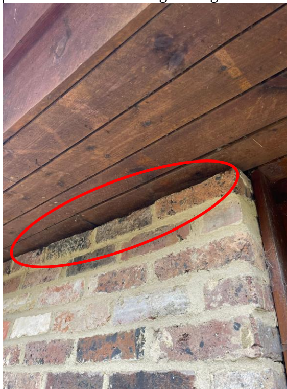
Photograph 15: Gap between soffits and wall.
