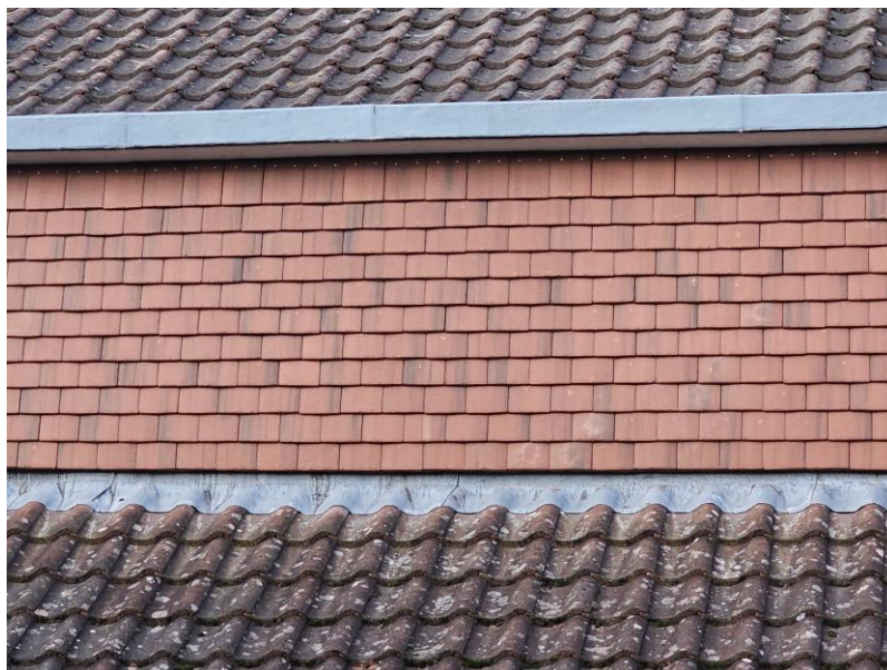
Photograph 5: Condition of the hanging tiles and associated lead flashings
