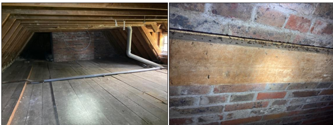
Photographs 7a (left) and 7b (right). 7a) View of the loft space access, view of the beams located to the top of the image. Image taken from the north facing south. 7b) View of a beam located to the rear wall (south of loft space) with several bat droppings identified.
