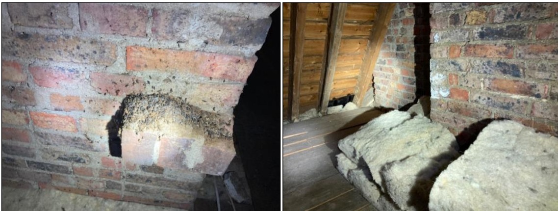
Photographs 9a (left) and 9b (right). 9a) View of a large number of bat droppings located to the southern aspect of the northern most chimney within this loft space, the photograph illustrates a large pile up on droppings on top of the exposed brick feature indicating more long-term use of this loft space. 9b) View of a chimney to the right of the image, and rafters and cladding located to the left of the image, the condition of the cladding and rafters is consistent to this throughout the void space.
