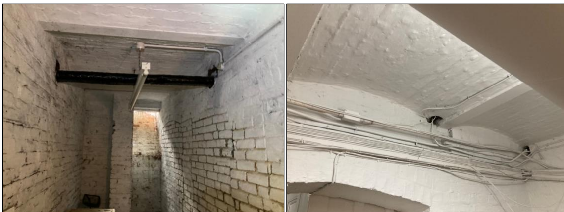
Photographs 6a (left) and 6b (right). 6a) View of a corridor space within the cellar/basement level with view of the access adjacent to the external ground floor gully that may act as possible access/egress to this area. 6b) view of hole with cables running through the first cellar room shown in photograph 5a.
