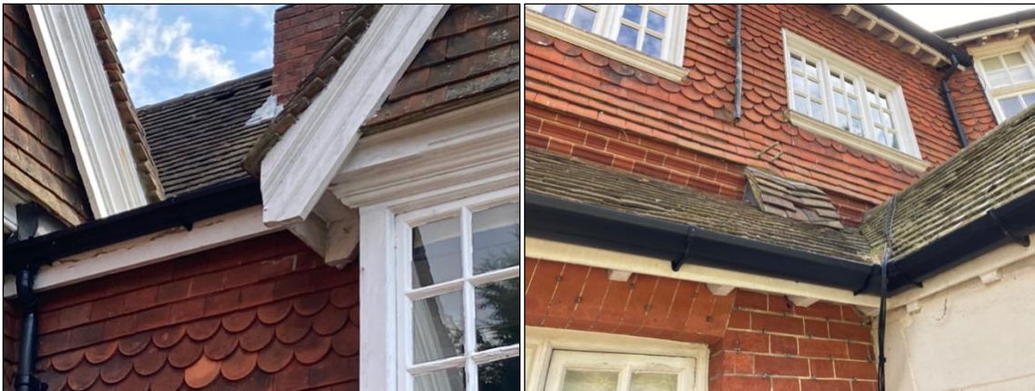
Photographs 3a (left) and 3b (right). 3a) View of lifted lead flashing and roof tiles noted to the western aspect of the property. 3b) View of lifted hanging and roof tiles noted to the northwestern aspect of the property.
