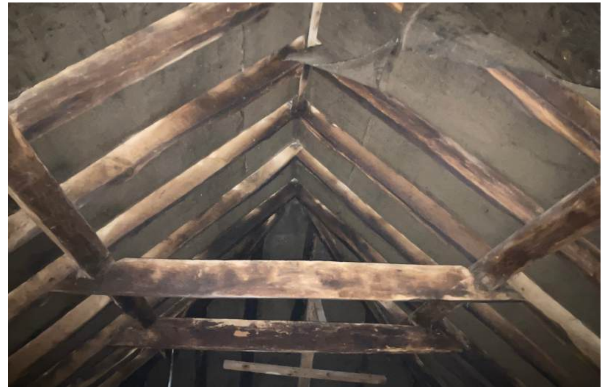
Sooted roof structure over former brewhouse/washhouse.
