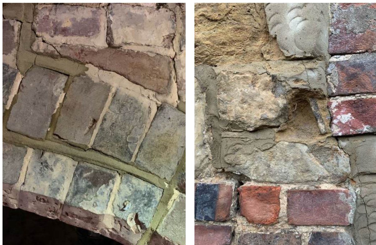
Examples of fireplace areas that need repairing.
