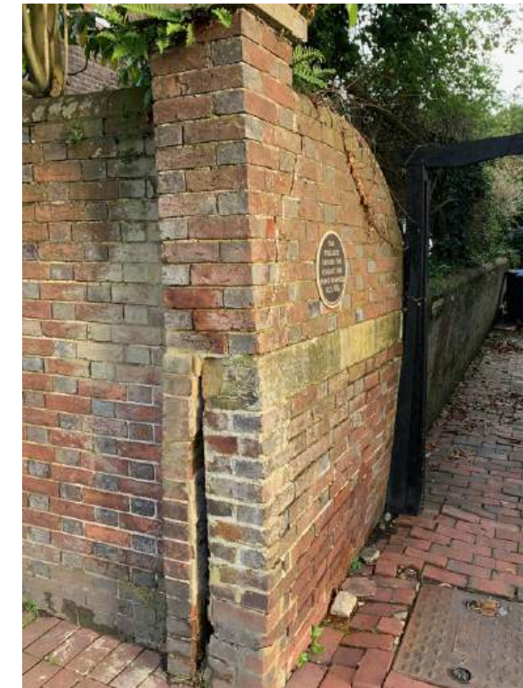
Damaged wall to be rebuilt.
