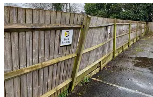
Area of damaged fence to the south
