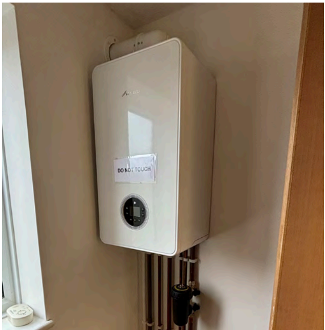
Gas boiler, ground floor
