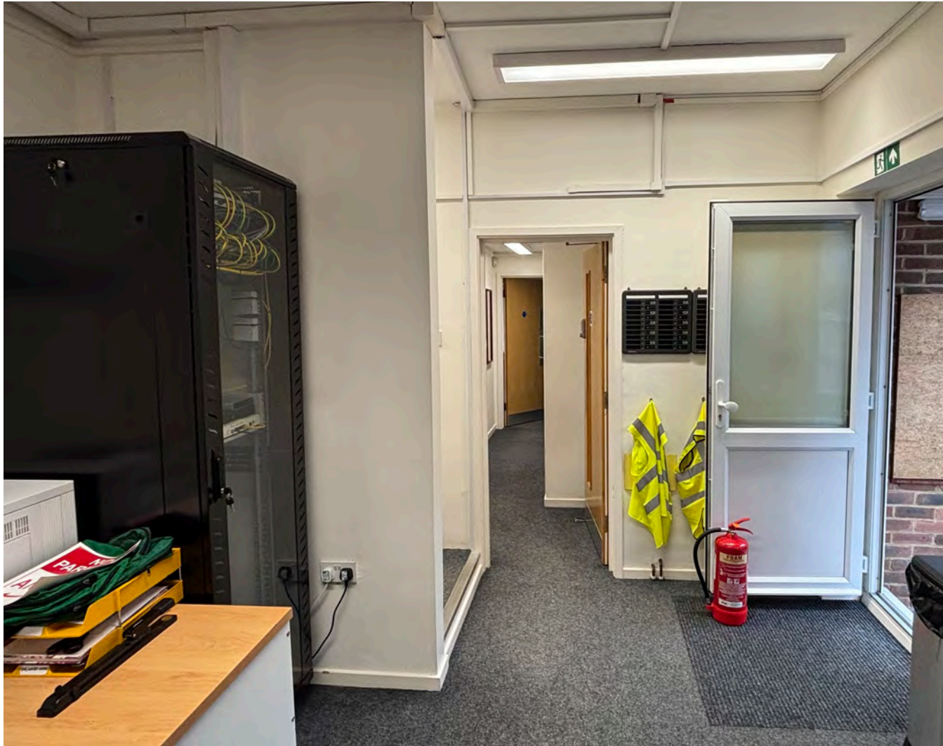
Excessive surface mounted services in the hall
