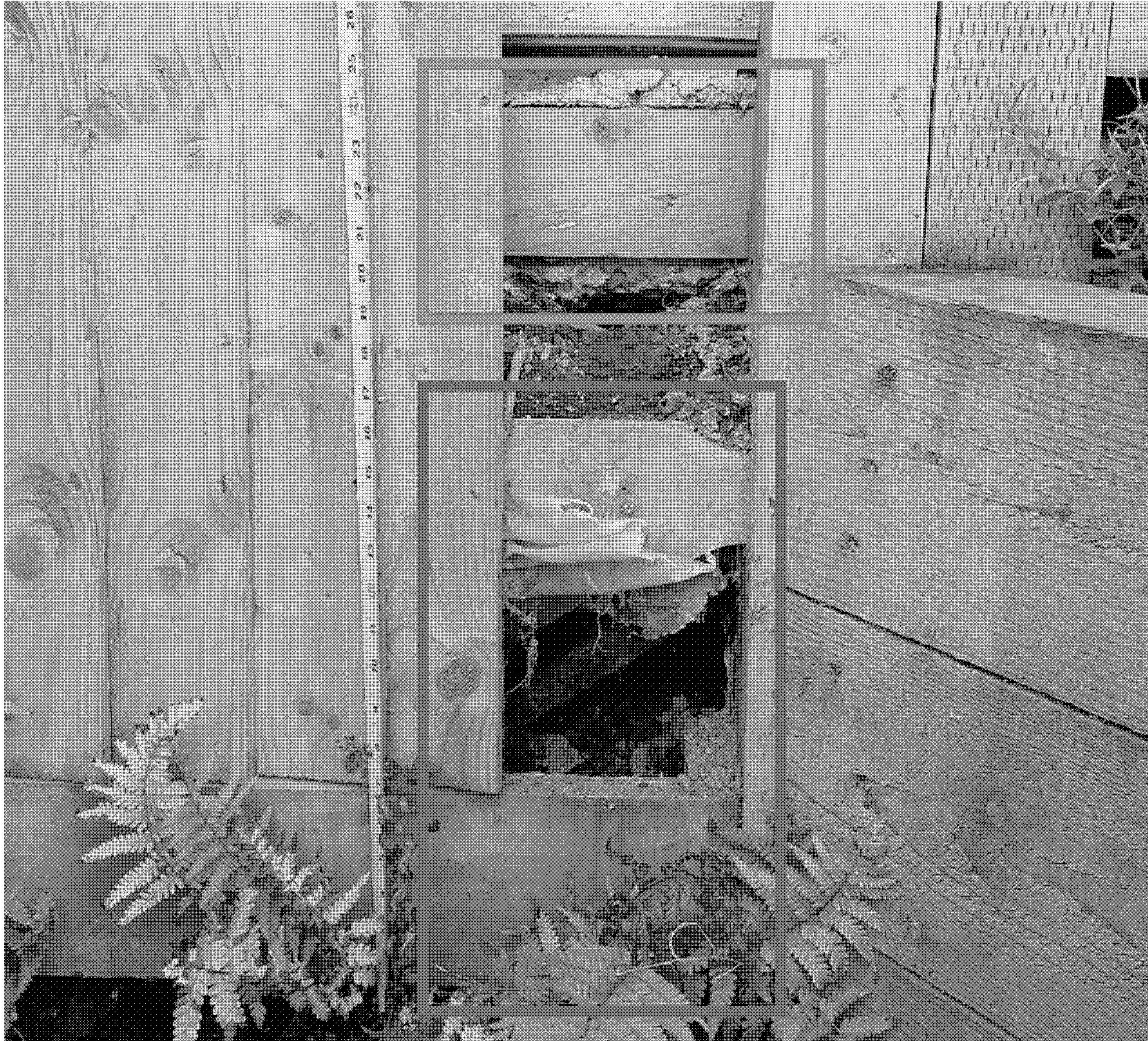
Figure 3: Original parts of the fence (outlined in blue) and the horizontal board that has been fixed to the back of the fence (red)
