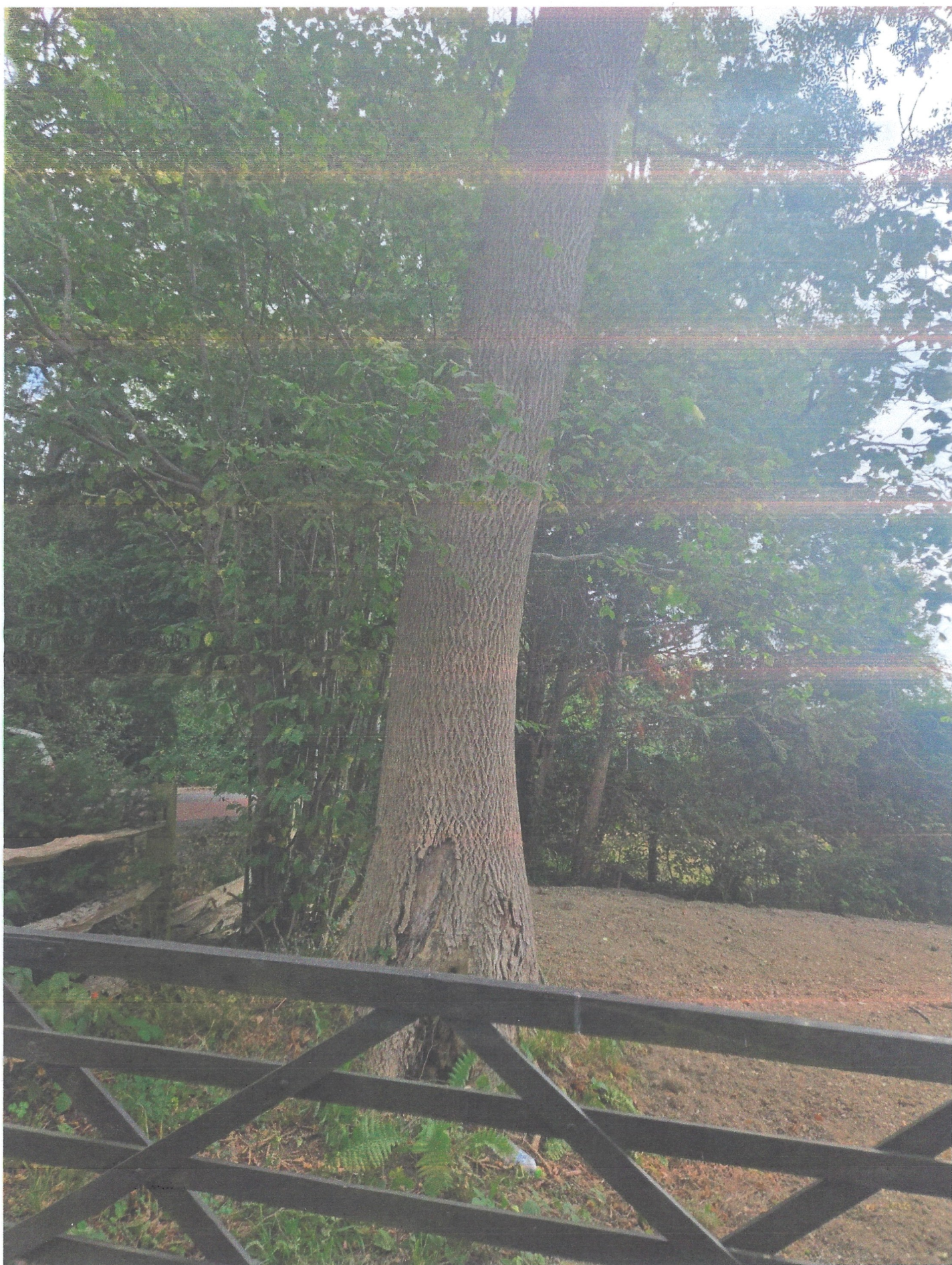
Tree over hanging Not fully shown But Branches over hanging main Road & the property.
