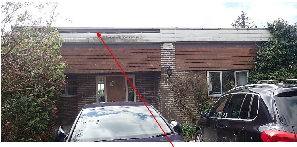
Fig. 4 – Front (N) view of house, showing missing UPVC fascia board
