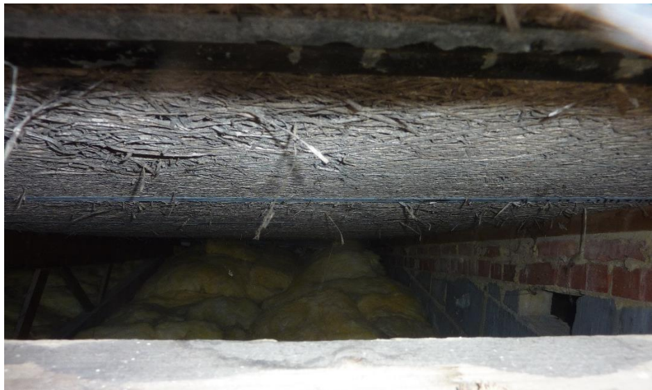
Fig. 5 – Shallow void behind recently lost fascia board, N side
