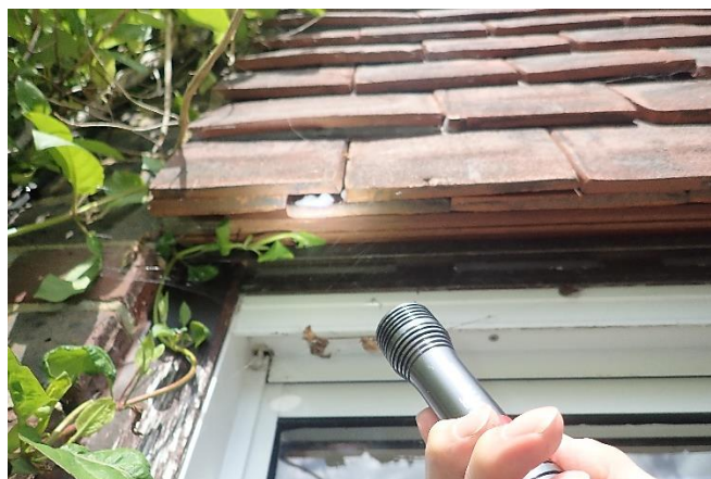
Fig. 6 – Small gaps between vertical tiles, S side, sealed with silicon by previous owner
