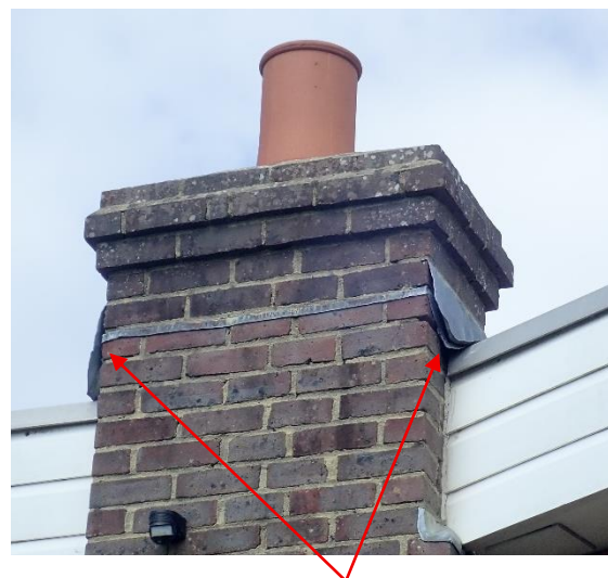
Fig. 8 - Small gaps beneath lead flashing, S side
