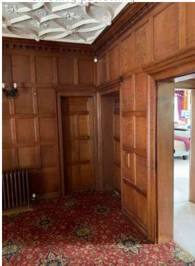
E Existing door to bedroom 4 locked shut (but retained insitu)
