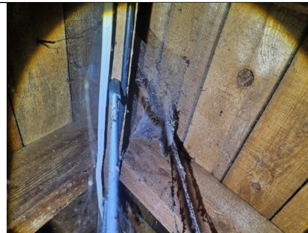
Figure 75: Bat droppings caught within a web above the pipe.
