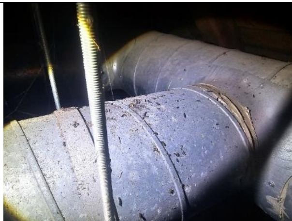
Figure 74: Droppings located ontop of the pipe within the loft space.
