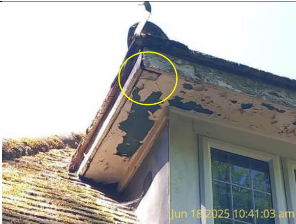
Figure 12: B2 – dormer window. There are gaps in the timbers of the dormers. These gaps provide suitable roosting features for bats.
