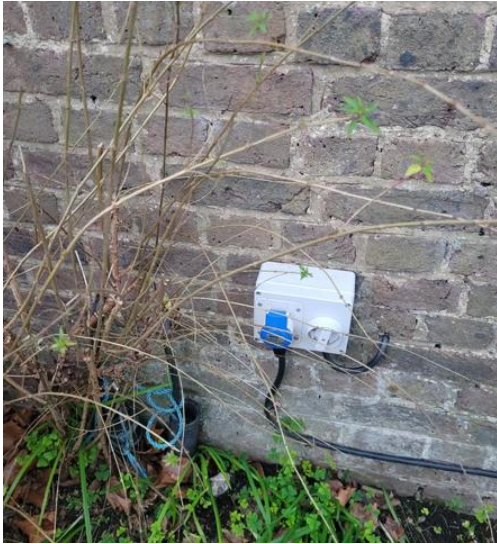
Photo 4: Existing utilises entering the Standen Farmhouse.
