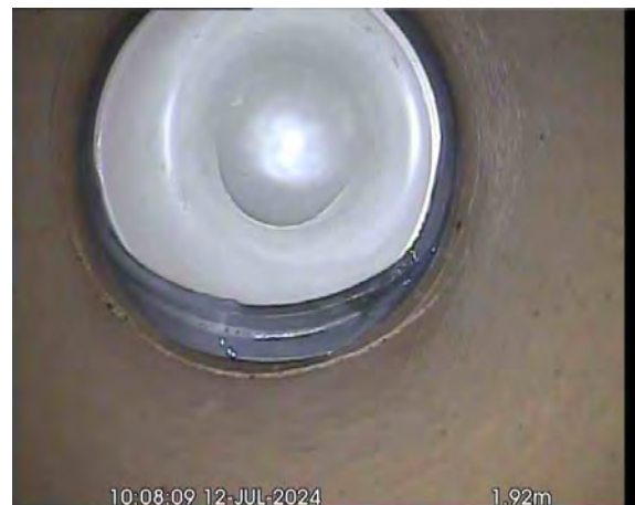
W_CX_dc0dc9d8-5d35-437e-89b2-f803bfeb8fe8_20240725_090809_548.jpg, 00:01:01, 1.92 m Sealing ring intruding, intruding but not hanging from 4 o'clock to 8 o'clock, (ON PAN CONNECTOR)
