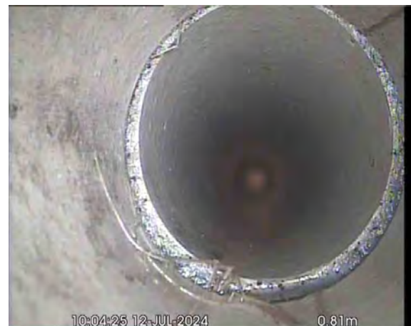
GULLYX_497c7feb-53ee-44b1-89dc-872bd2b7a9cf_20240725_090218_006.jpg, 00:01:01, 0.81 m Roots, fine at joint
