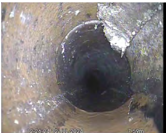
MH5X_a25c901e-431c-4751-af44-e6286baac714_20240725_094843_842.jpg, 00:01:51, 7.59 m Attached deposits, grease from 12 o'clock to 5 o'clock, 5% cross-sectional area loss
