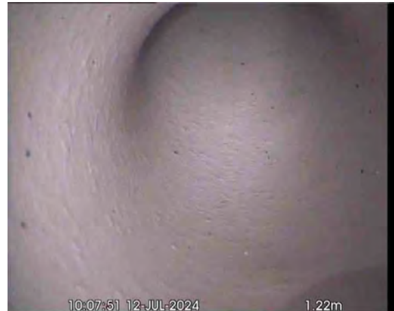
W_CX_e67dc308-cdad-4b4f-8f22-12bae3fd920a_20240725_090718_061.jpg, 00:00:43, 1.22 m Line deviates up, REST BEND
