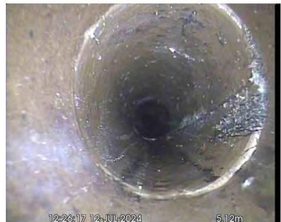
MH5X_109efa46-164d-464f-96dd-18bcad47188e_20240725_094816_811.jpg, 00:01:44, 5.12 m Roots, fine at joint
