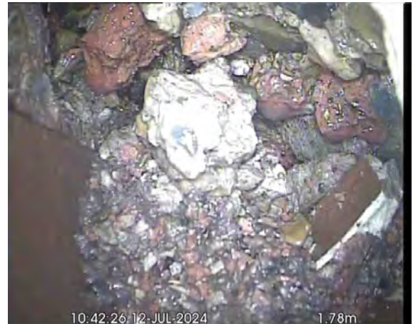
REDUNDANTX_8ff2f762-c2e0-455c-bf22-40405fb29865_202 40725_091223_724.jpg, 00:00:56, 1.78 m Survey abandoned, S/A - REDUNDANT LINE
