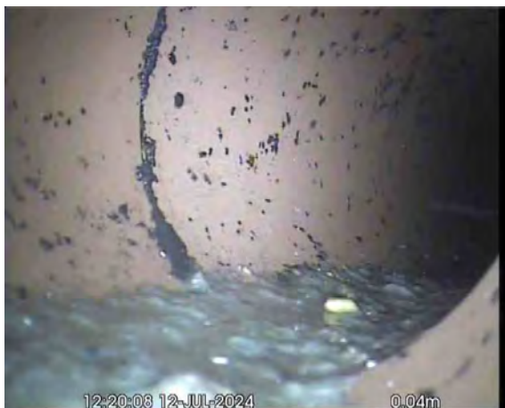
CAPPED OFFX_80832dd5-8ef6-4f5d-89c0-115ac1b2d810_20240725_094214_228.jpg, 00:00:41, 0.04 m Line deviates right
