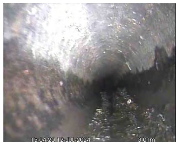
MANHOLEX_9f739453-0b6d-4c3b-aa2f-970cef82bb99_20240725_102213_871.jpg, 00:00:51, 3.01 m Settled deposits, fine, 5% cross-sectional area loss
