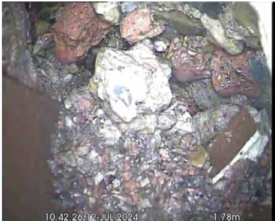
REDUNDANTX_716789ca-25ee-4cc2-8135-a7bc7aff19d4_20 240725_091212_524.jpg, 00:00:56, 1.78 m Settled deposits, hard or compacted, 100% cross-sectional area loss
