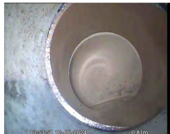
SVPX_6dc84003-04ba-4f4b-a2bc-ade636d85d44_20240725_095258_153.jpg, 00:00:43, 0.81 m Material changes to polyvinyl chloride
