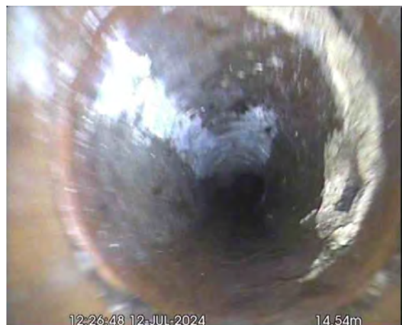
MH5X_b9529b71-08d6-4df3-a0ef-83327201d51f_20240725_094926_931.jpg, 00:02:15, 14.54 m Hole in drain or sewer at 4 o'clock
