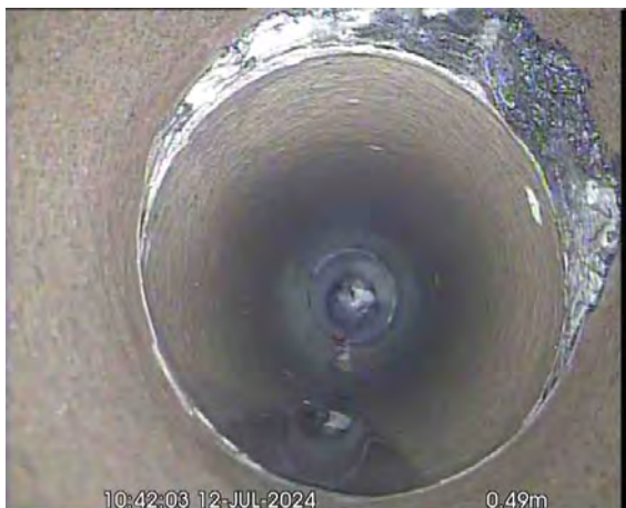
REDUNDANTX_0df9520d-4cc8-45ca-b8b9-6ea8c8cc1138_20 240725_091130_965.jpg, 00:00:34, 0.49 m Joint displaced, large
