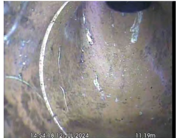
RWDPX_86dc6ebb-da85-45a0-a40c-1b8118d31bb7_20240725_101744_768.jpg, 00:01:49, 11.19 m Line deviates up, REST BEND
