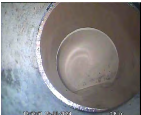
SVPX_6126ff3a-8feb-42cf-b4a8-289a35627abd_20240725_095243_344.jpg, 00:00:43, 0.81 m Joint displaced, medium
