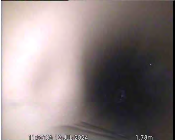
MH2X_63ec8ede-2157-460a-bba6-3a2739af30ac_20240725_093101_292.jpg, 00:01:11, 1.78 m Water level, 5% of the vertical dimension
