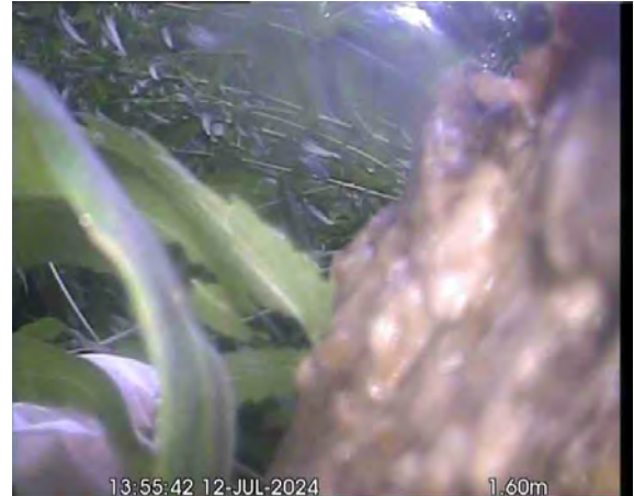
SVPX_9d8768b1-86dd-4d7b-b136-613c52434c58_20240725_095530_137.jpg, 00:01:28, 1.60 m Survey abandoned, S/A - OPEN PIPE - SOIL VENT PIPE NOT CONNECTED UP
