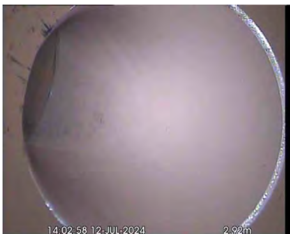
GULLYX_0fb9ef59-34cb-4c01-8650-9407a85952f5_20240725_101359_633.jpg, 00:01:09, 2.92 m Line deviates left
