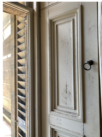
Example of timber shutter requiring restoration
