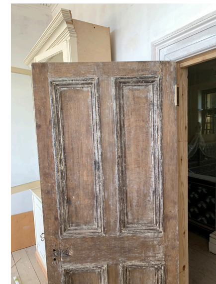
Example of door restoration and decoration required
