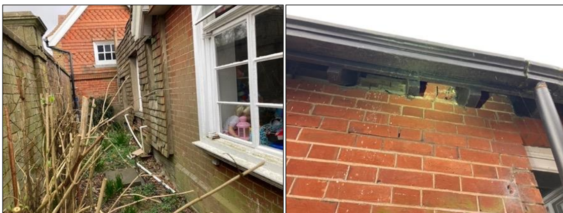
Photographs 3a (left) and 3b (right). 3a) View of the western aspect of the cottage with view of the close proximity of the building and the adjacent boundary wall. View of the garage aspect is noted to the top of the image. 3b) View of the gaps noted to gables on the western aspect of the cottage.
