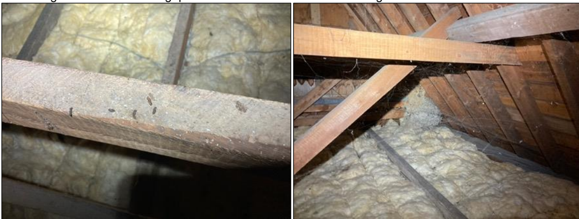
Photographs 5a (left) and 5b (right). 5a) View of bat droppings located along one of the collar ties within void 1. 5b) View of the collar tie within void 1 with a large disused wasps nest located to the far right of the image.
