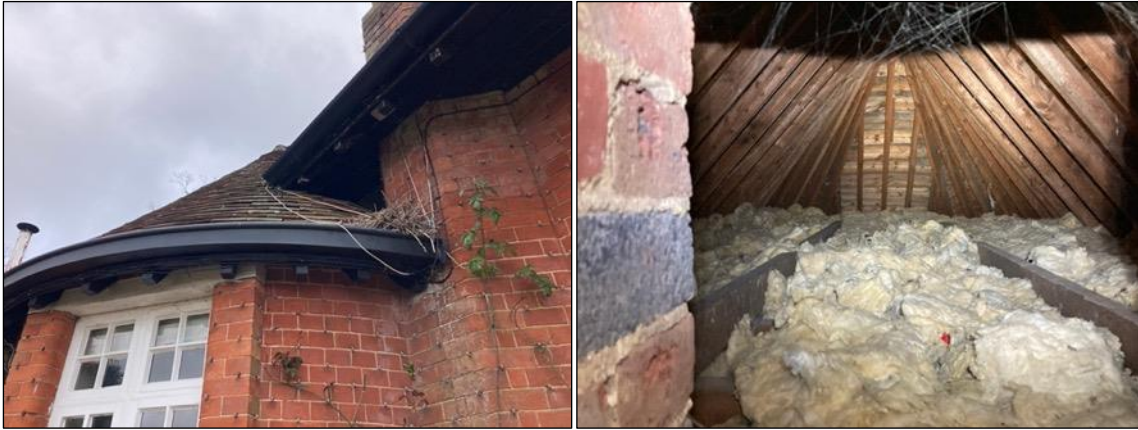
Photographs 7a (left) and 7b (right). 7a) View of the exterior of tower 1 as taken from the eastern aspect with view of lifted tiles noted to the center of the image and bird nesting material to bottom right of the towers roof. 7b) Interior view of the towers void as taken from the hole noted in void 2 (photograph 6a).
