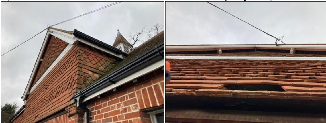
Photographs 8a (left) and 8b (right). 8a) exterior view of the garage block with the image taken from the eastern aspect, large sections of hanging tiles noted to this feature with view of missing/lifted tiles noted. 8b) view of the missing tiles taken from the base of the southernmost garage block with the missing tiles noted to the centre of the image visible in photograph 8a.
