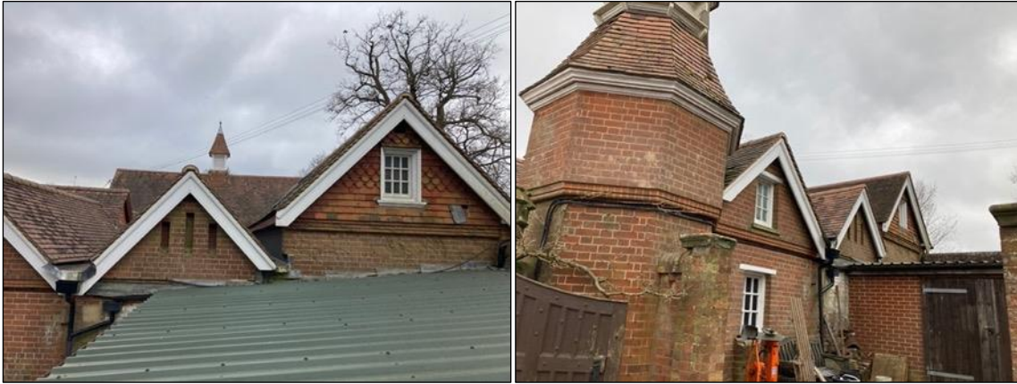
Photographs 10a(left) and 10b (right). 10a) View of the stores from the northern aspect with view of damaged hanging tiles to the right of the image and well-kept roof tiles across the image. 10b) view of the stores as taken from the eastern aspect of the site with a view of tower 2 located to the far right of the image.
