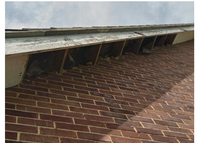
Bottom of the soffit box missing on the south elevation.
