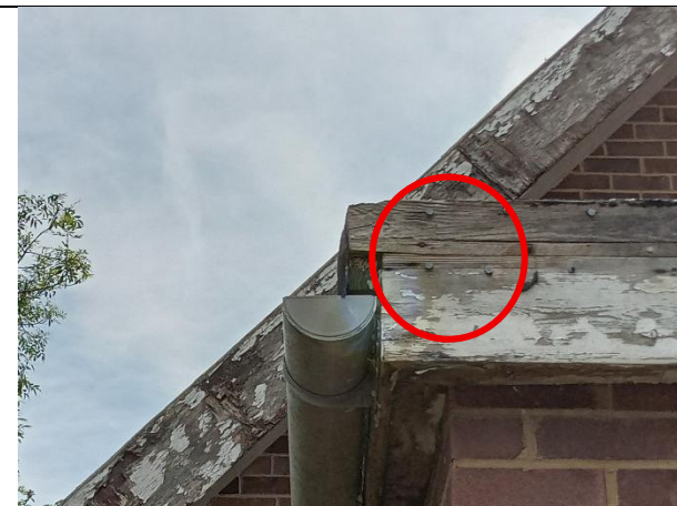
Hole in the soffit box on the north elevation.
