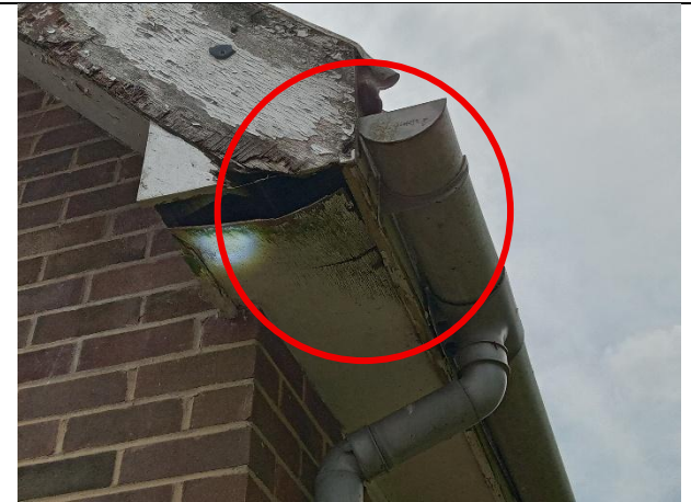
Hole in the soffit box on the east elevation.
