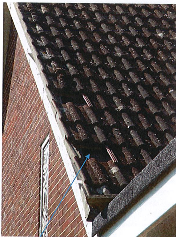
Missing tiles to southern gable Photograph C4
