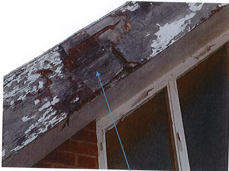
Wet rot to plywood barge board Photograph C10
