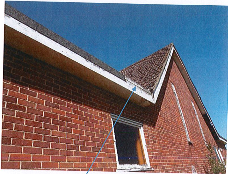
Missing section of felt covering to verge Photograph C9
