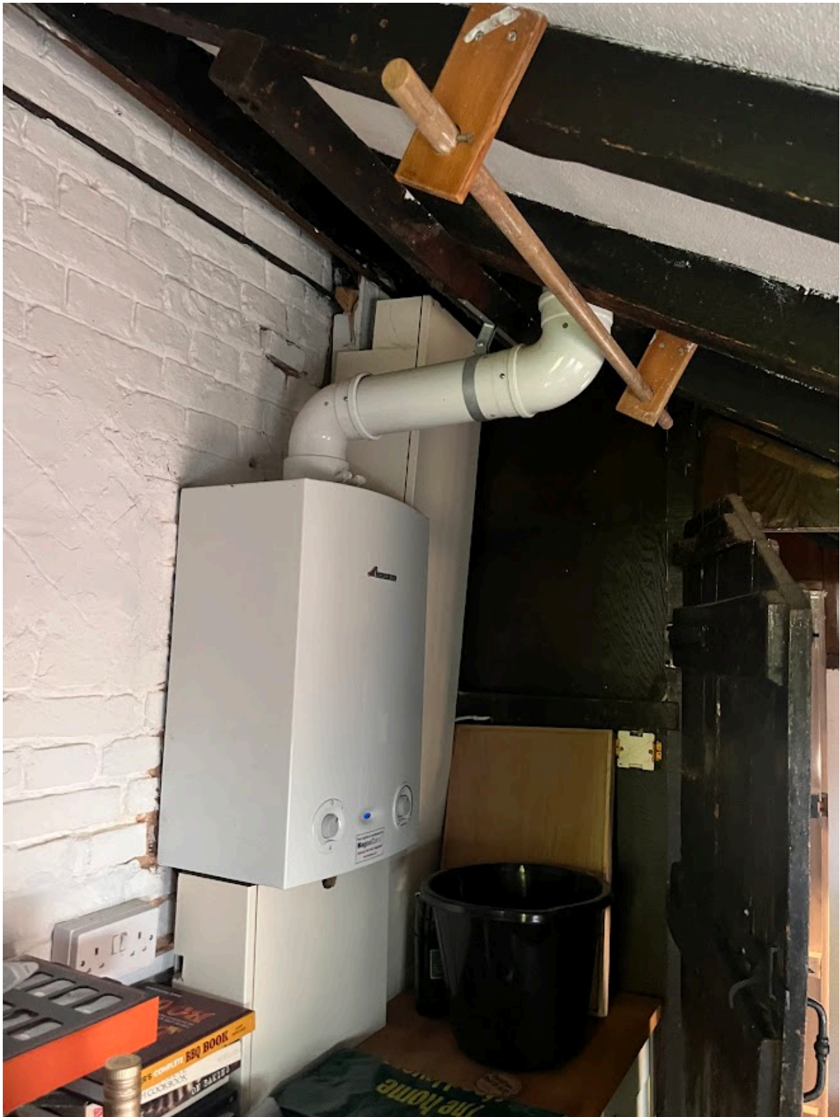
Boiler with venting flu
