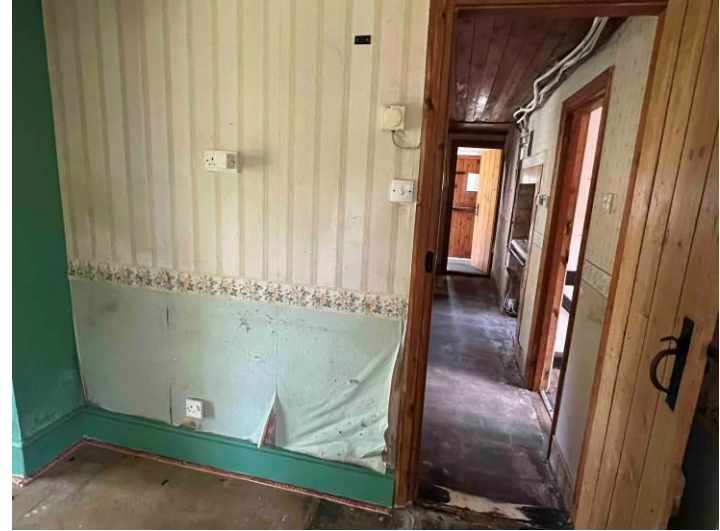
Poor state of interior
