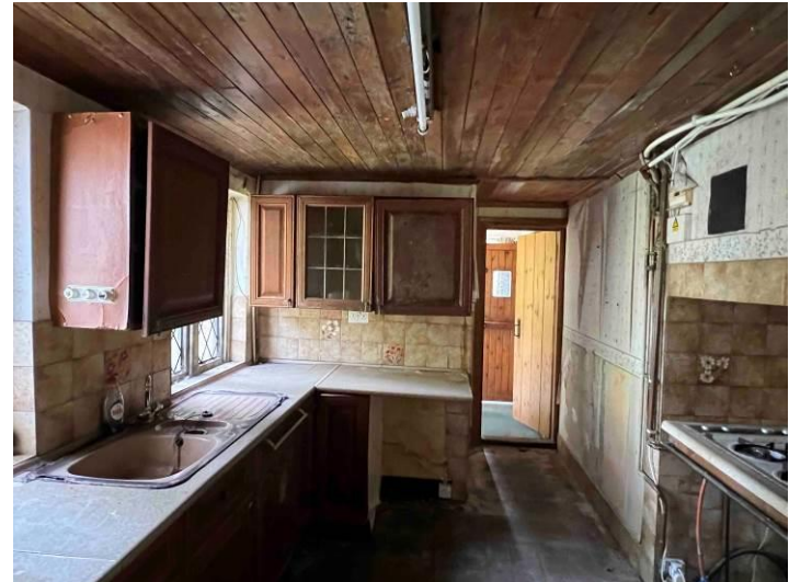
Dilapidated kitchen area
