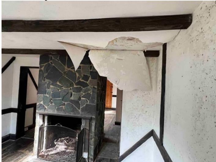
Dilapidated interior – ceiling collapse
