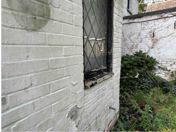
Dilapidated widow and exterior wall
