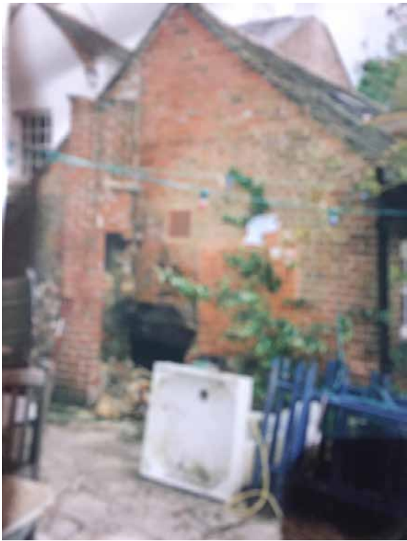
Photograph provided by Gina Nichols- previous owner. Condition of Bakehouse around 1990 - damaged brickwork and holes in the walls, partially demolished chimney stack and missing chimney pot. The photograph demonstrates historically poor condition of the building.
