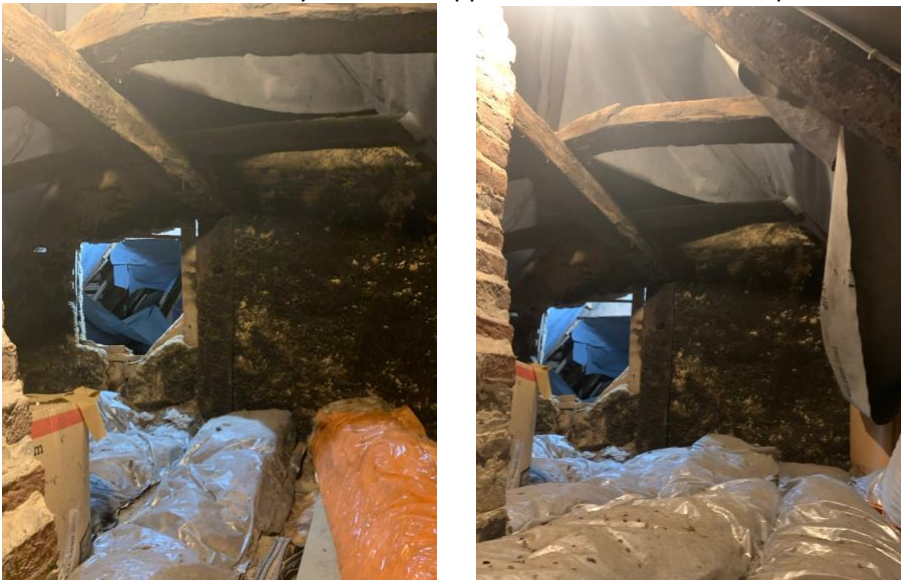
Partition at C-C with a breach through. The collar purlin is present with collars above, one of which is broken. The collar purlin runs into the crown post. Down braces are visible.
