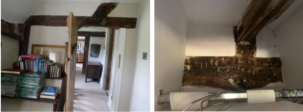
North side of partition C-C where the cross-beam runs through the stud partition which sees the middle bedroom intrude into the service chamber.
