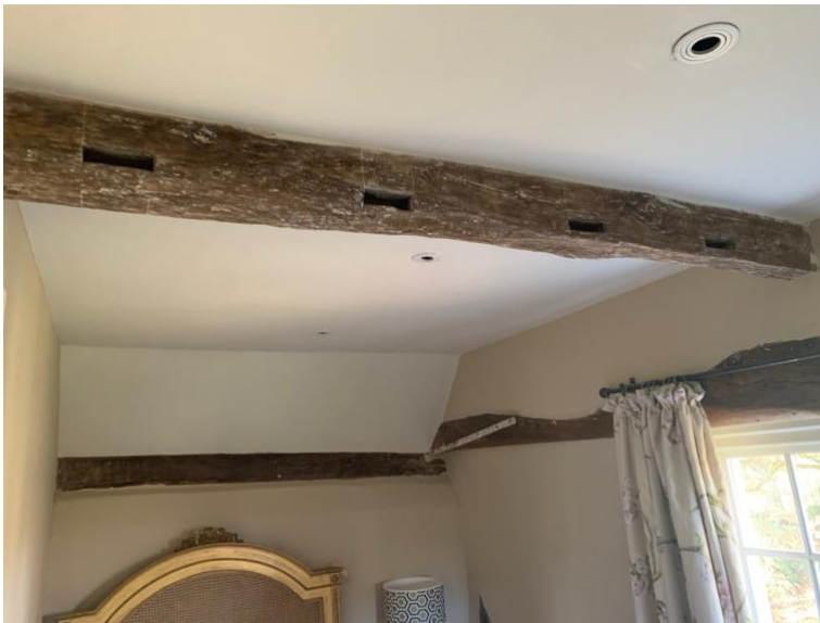
Altered north end service chamber which and along with the service bay to the ground floor, stairs, east wall, and hall chamber, has seen extensive change.
