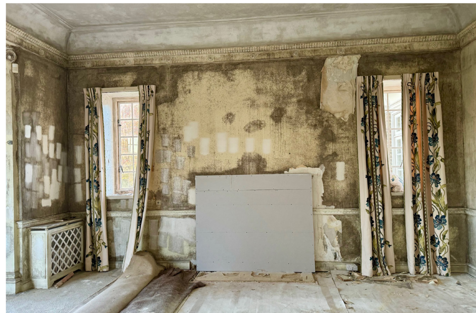
Top Left: Significant moisture degradation is evident to all surface
