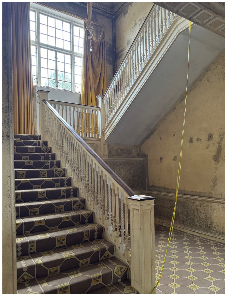
Above: The main staircase. Moisture damage is evident to all walls
