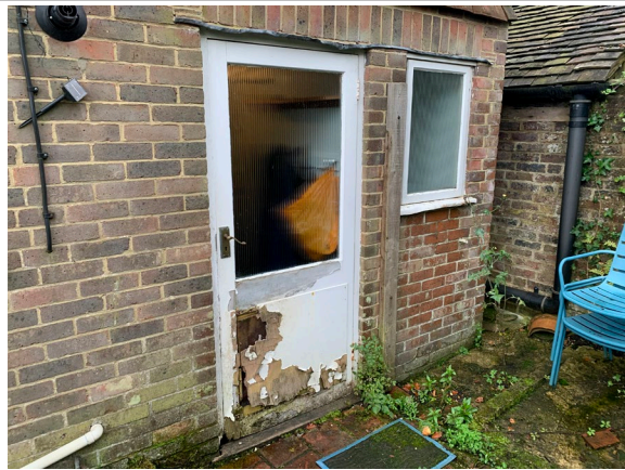
Image of rotten and damaged door to the side extension
