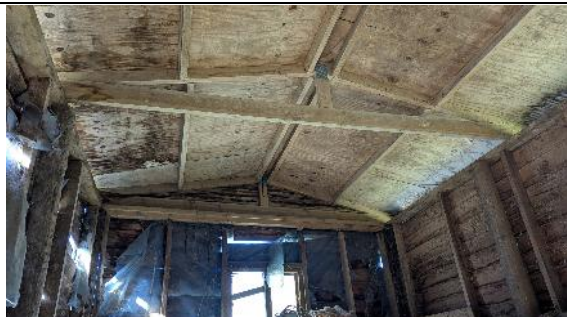
Photo 5: The roof and interior of the barn facing west, showing wooden cladded walls, some of which were cover in plastic sheeting.
