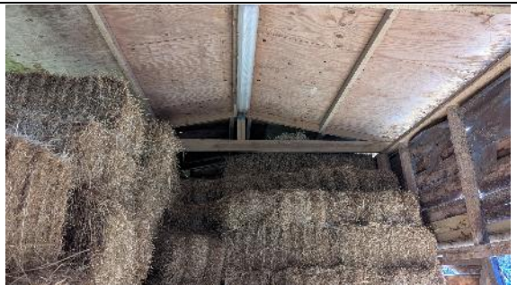
Photo 6: The roof and interior of the barn facing west, showing wooden cladded walls and the stored hay bales.
