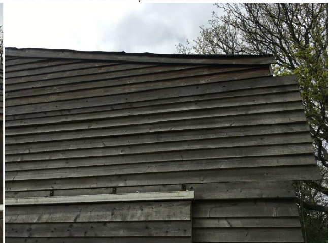
Eastern face of building, gaps in weather boarding
