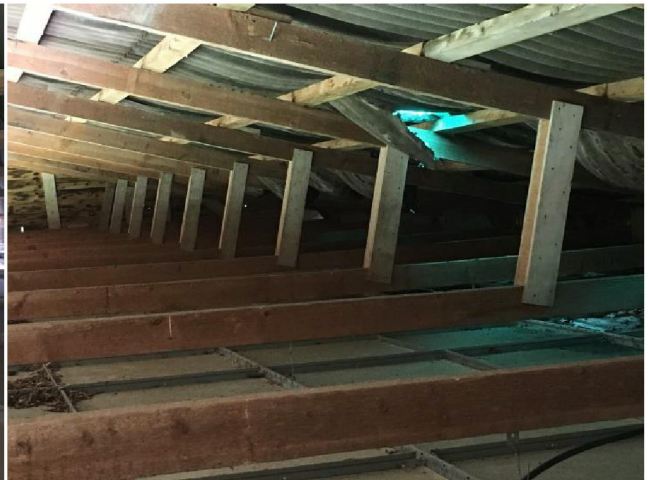
Broken roof panelling
