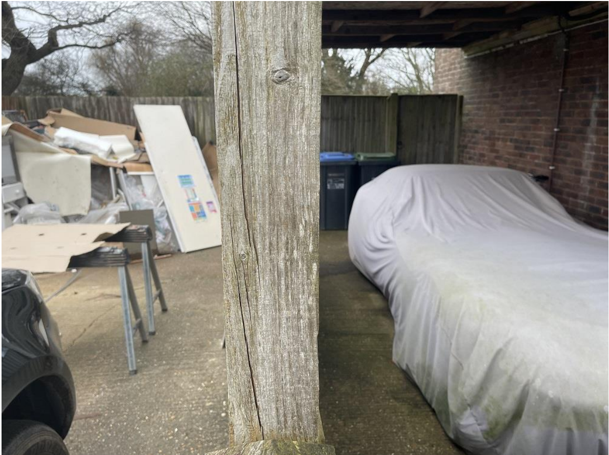
View in to existing car port and adjoining parking area of load bearing concrete slabs.
