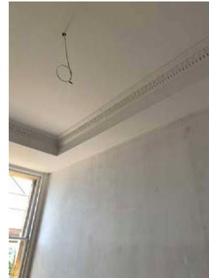
Example of ventilation dropped ceiling with cornicing
