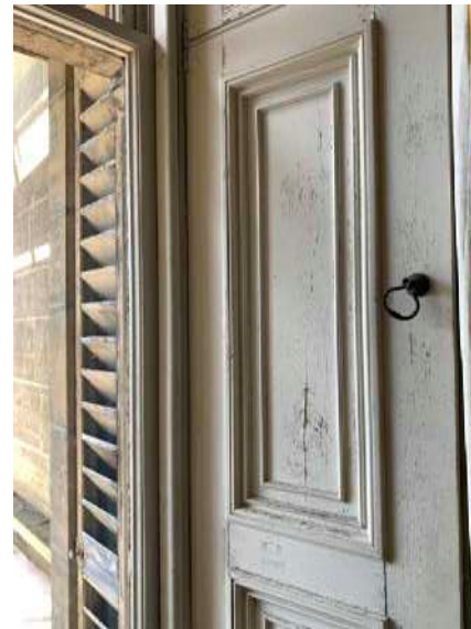
Example of timber shutter requiring restoration
