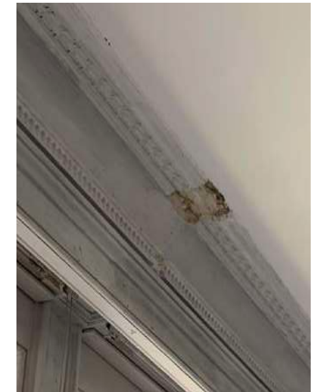
Example of repair required following removal of non original wall
