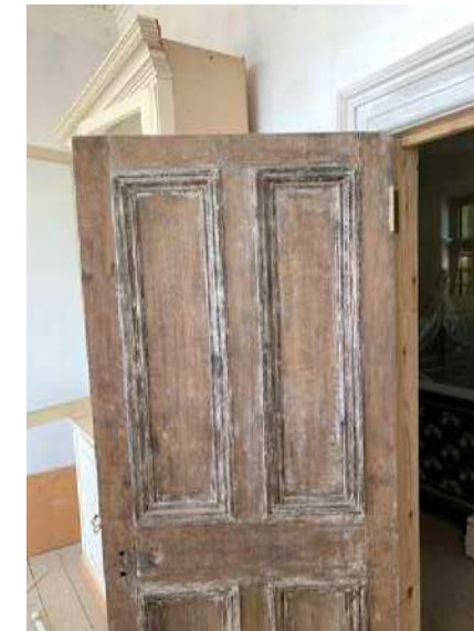
Example of door restoration and decoration required
