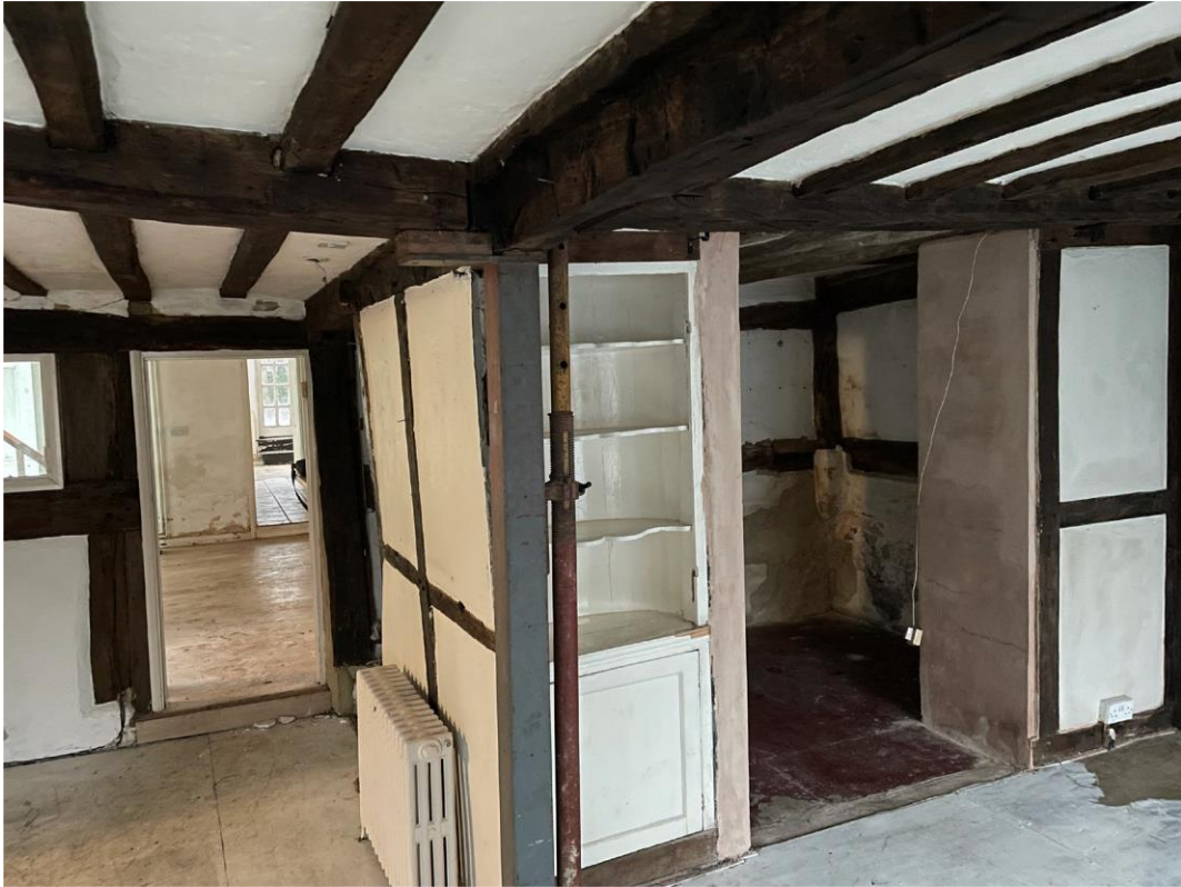
Figure 14: Central supporting post to main living room. Source: McCarey Simmonds, Structural Inspection Report of 15 th March 2023
