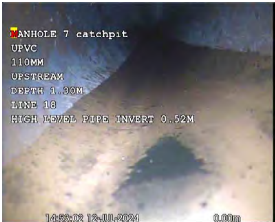
RWDPX_21485e2f-4097-497f-806e-9df9c5496cab_20240725_101604_864.jpg, 00:00:33, 0.00 m Start node, catchpit, reference: MANHOLE 7 (MH7) - CATCHPIT (CP), (HIGH LEVEL PIPE - INVERT - 0.52M)
