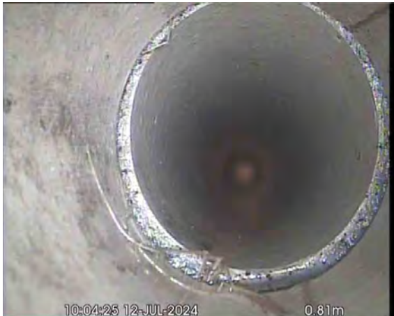
GULLYX_be408751-b267-4dcb-87b2-47920da53df0_20240725_090226_317.jpg, 00:01:01, 0.81 m Joint displaced, medium
