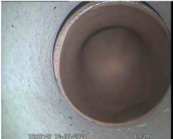
W_CX_1865770f-a7a0-438a-95c3-9da68d53db4d_20240725_090701_492.jpg, 00:00:39, 1.13 m Joint displaced, medium
