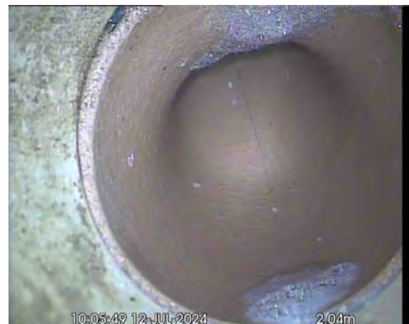
W_CX_96eda4f4-1bbb-49c3-bdf5-b6f3418d49e6_20240725_090429_528.jpg, 00:00:47, 2.04 m Line deviates up, REST BEND
