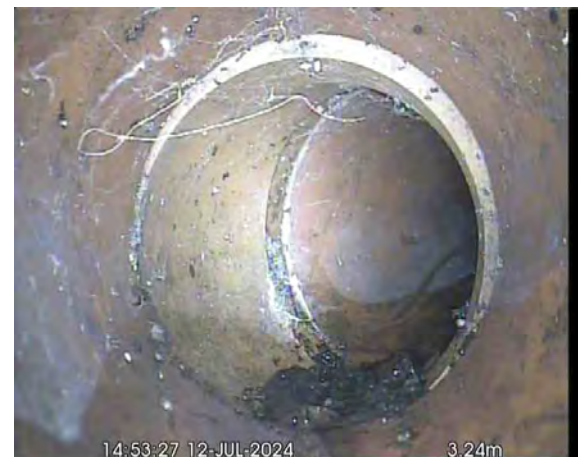
RWDPX_b04b44a7-7c3f-4146-a3f3-0906ec81aae0_20240725_101714_425.jpg, 00:00:58, 3.24 m Line deviates right
