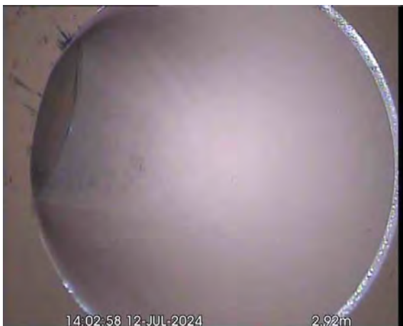
GULLYX_0fb9ef59-34cb-4c01-8650-9407a85952f5_20240725_101359_633.jpg, 00:01:09, 2.92 m Line deviates left
