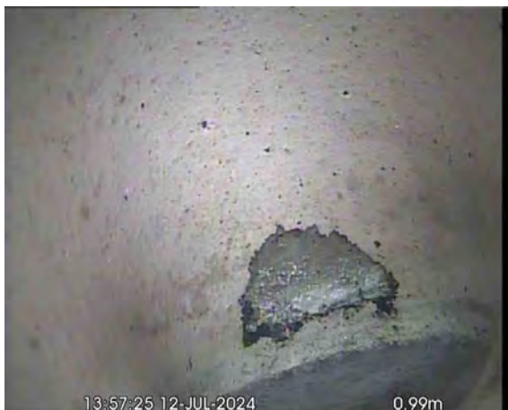
GULLYX_6d63e6bc-a192-46ee-bb28-5b54a1a3e0d8_20240725_095748_794.jpg, 00:00:39, 0.99 m Finish node, gully, reference: GULLY
