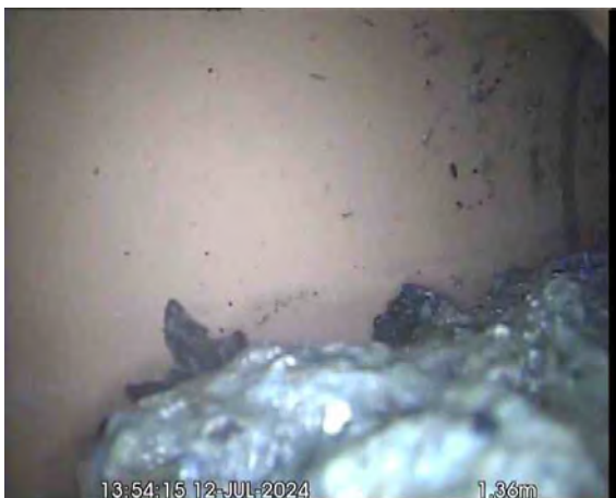
SVPX_b8b7fa38-33f3-45aa-a30b-8dfd9bcbd768_20240725_095417_154.jpg, 00:01:07, 1.36 m Settled deposits, hard or compacted, 15% cross-sectional area loss
