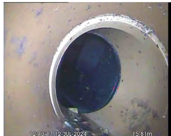
MH4X_9d8f4504-f323-432b-9698-14d451cd618f_20240725_094016_482.jpg, 00:01:29, 15.81 m Line deviates left
