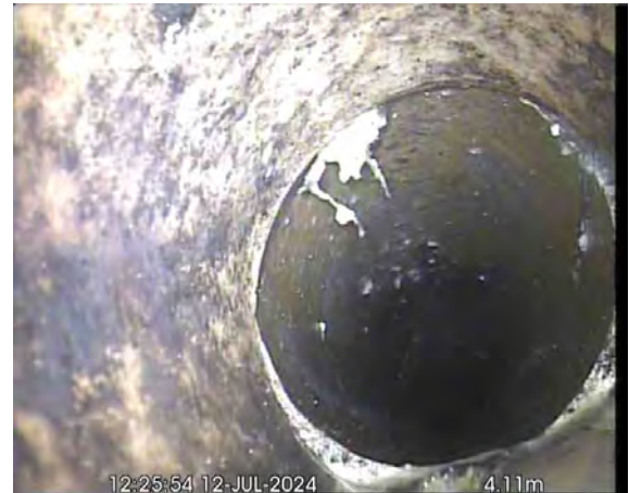
MH5X_059f6707-2778-4d9f-998a-3e91e87c5d40_20240725_094727_709.jpg, 00:01:24, 4.11 m Joint displaced, medium
