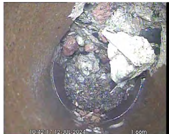
REDUNDANTX_29814b43-2bf2-411c-83a3-7448b2e32080_2 0240725_091151_156.jpg, 00:00:47, 1.66 m Broken pipe from 10 o'clock to 3 o'clock
