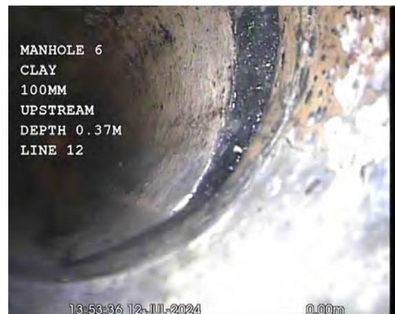
SVPX_74d44b96-72da-442c-8602-c87605640ac0_20240725_095222_464.jpg, 00:00:28, 0.00 m Water level, 0% of the vertical dimension
