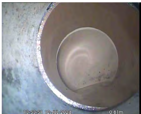
SVPX_6126ff3a-8feb-42cf-b4a8-289a35627abd_20240725_095243_344.jpg, 00:00:43, 0.81 m Joint displaced, medium
