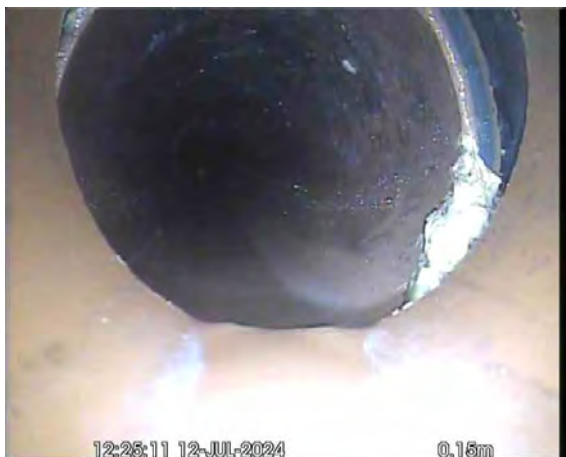
MH5X_a67b5490-9c73-459b-9229-8a05c12ea946_20240725_094558_658.jpg, 00:00:41, 0.15 m Joint displaced, large
