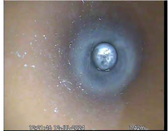
CAPPED OFFX_b9c4dbb3-d9c6-4d09-9f4f-e40713d124b7_20240725_0 94300_939.jpg, 00:02:19, 7.42 m Survey abandoned, S/A - CAPPED OFF
