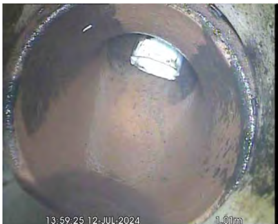
BASINX_40e5934f-6751-4c2f-8103-7d817af70ed0_20240725_101004_289.jpg, 00:00:28, 1.01 m Line deviates up, REST BEND
