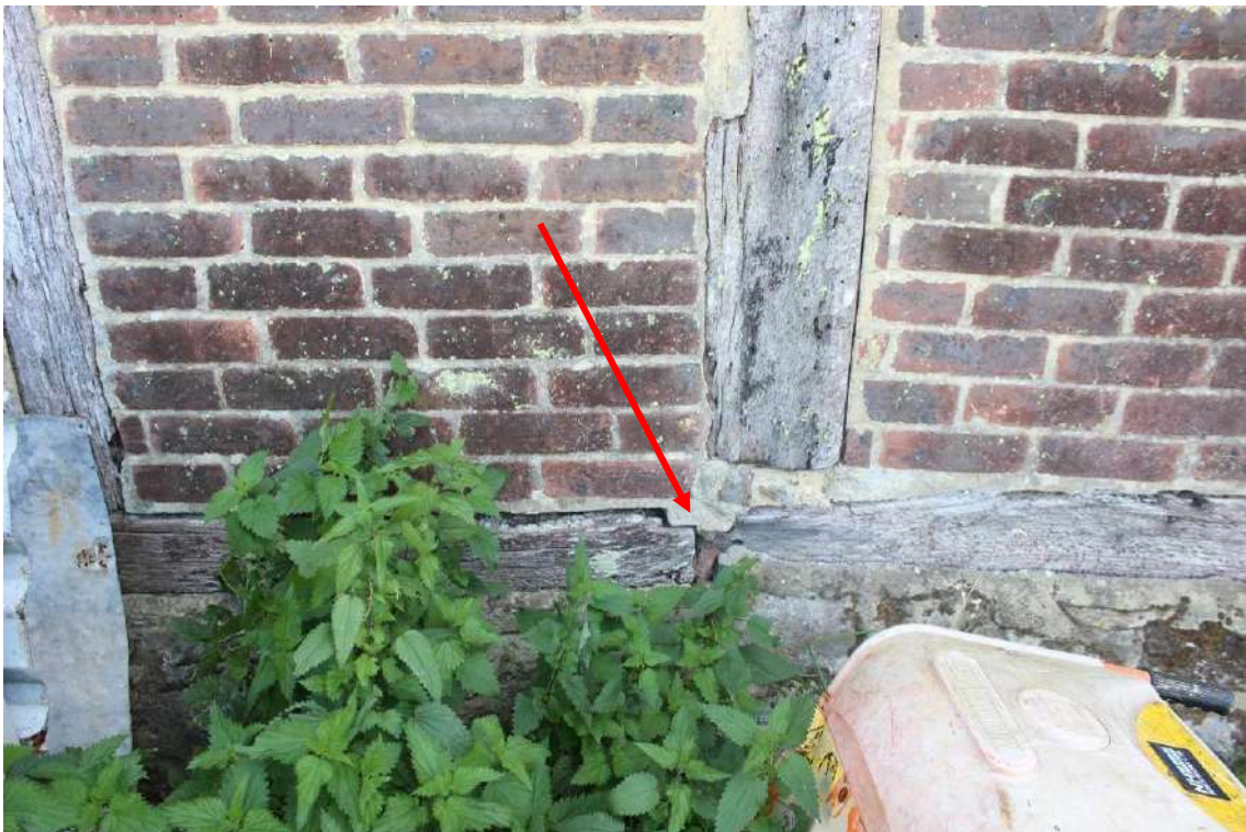
North elevation break in sill beam immediately east of post A1
