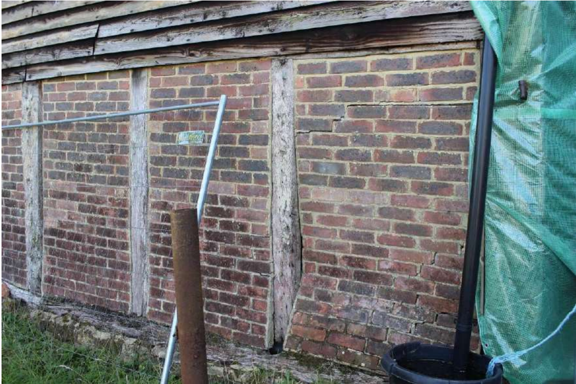
North wall with post C1 at right edge of image showing modern brick infill and stone plinth both with cementitious mortar
