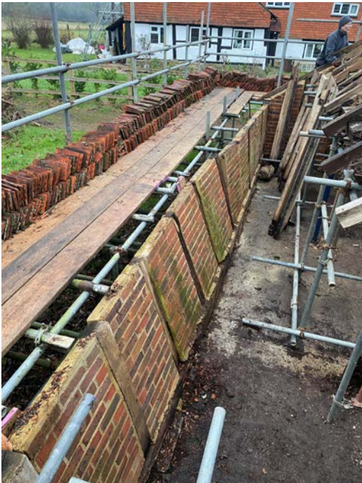
collapsed wall with roof removed
