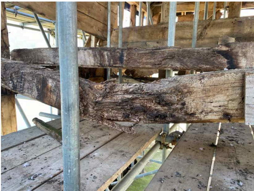
The photograph above shows the wet rot that is directly under the missing tiles that are apparent in the previous photograph. There are nine of these structural first floor beams missing, having been removed before the current ownership. Replacements have been ordered but cannot be installed until approval is gained from the planning authority.
