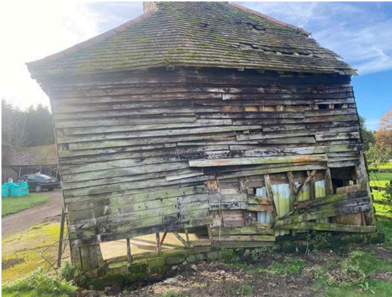
East face of granary before removal of tiles and cladding, showing lean to the south and some of the failed timbers.
