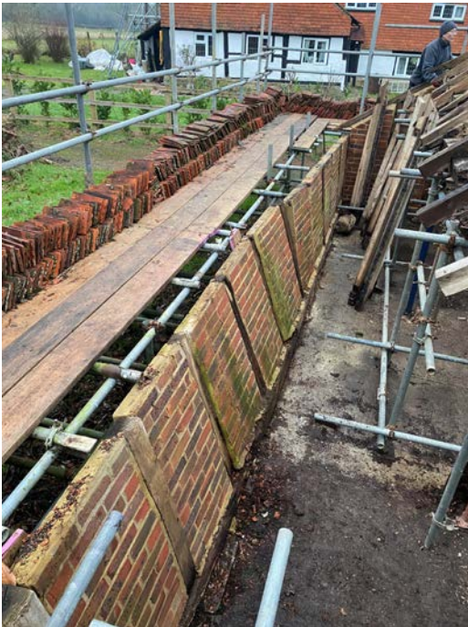
collapsed wall with roof removed
