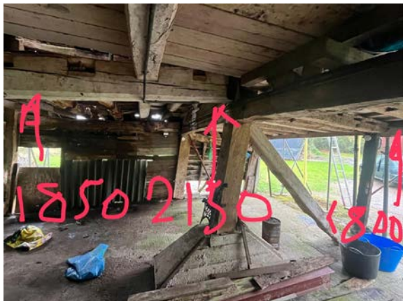
Central post with existing concrete flaunching and strut. (Note lean)
