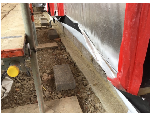
The outer brickwork was not in place to all plots noted above at the time of our inspection.
