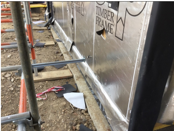
The outer brickwork was not in place to all plots noted above at the time of our inspection therefore MEC Environmental we're unable to inspect the membrane spanning the perimeter cavity walls.
