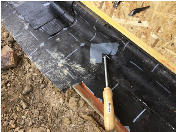
Weld defect found upon our inspection to plot 5.
