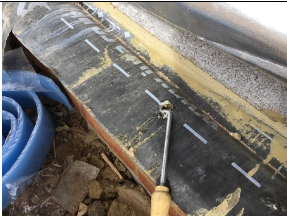
Hole found upon our inspection to plot 10.
