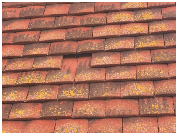
Occasional missing hanging tiles
