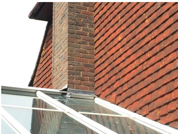
Lifted lead flashing at chimney join with conservatory
