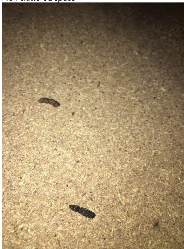
Bat droppings on top of water tank
