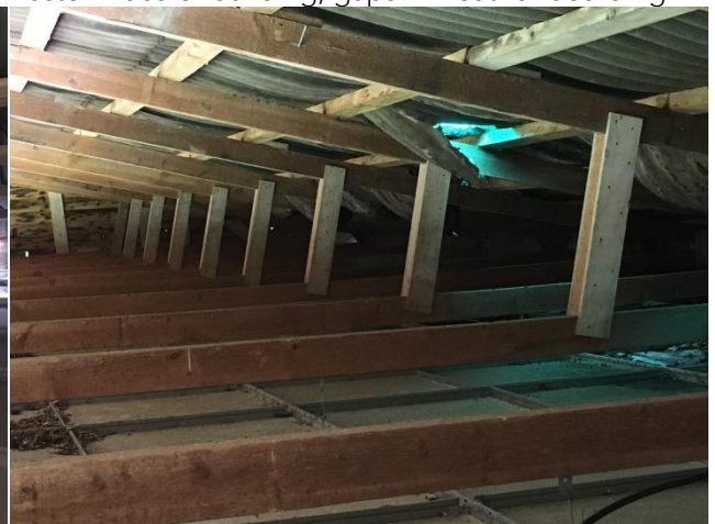
Broken roof panelling
