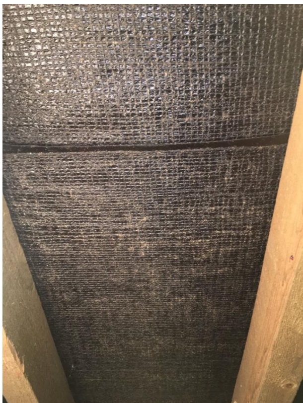
Tightly fitting lining
