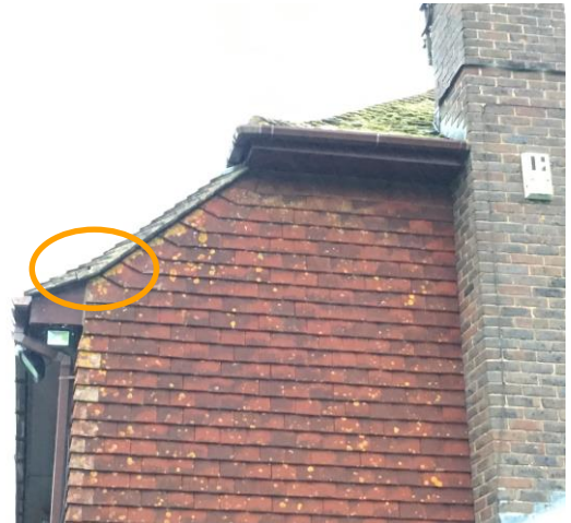
Survey 3 (B2): Point of re-entry at 06.11 on 12 September (missing mortar on edge of roof on south elevation, common pipistrelle x1).
