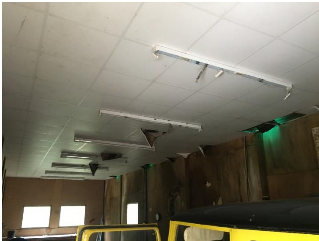
Internal space, peeling ceiling panels, light
