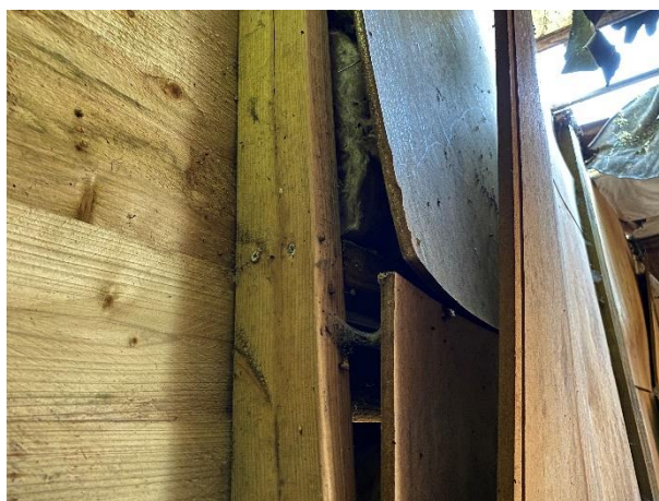
Photo 8: Lifted plasterboard showing cavity insulation
