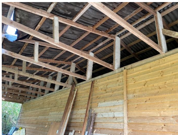
Photo 6: Large gap in wall on southern elevation
