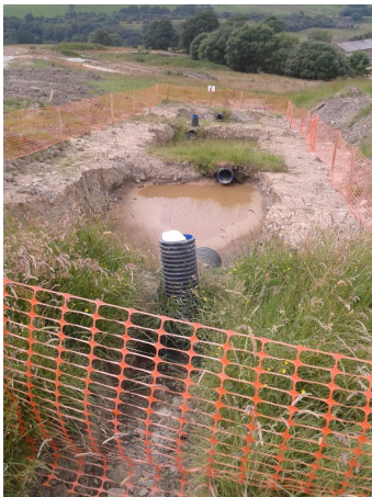
Figure 2: Settlement lagoon and flocculent station
