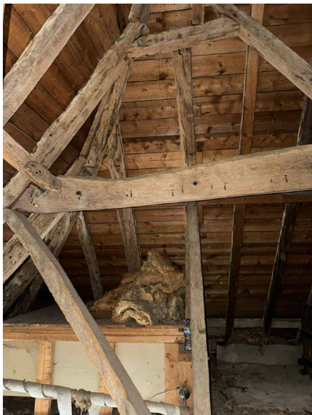
interior of north hip of C17th range showing sarking boards
