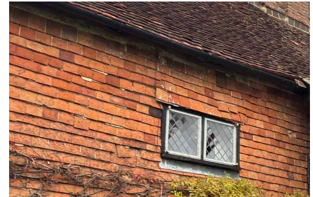
slipped and missing tiles present to southern elevation
